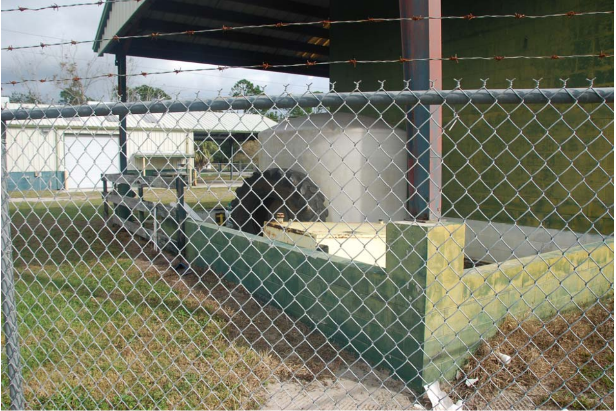
Photo 7: Close up of storage tank and containment, facing northeast
