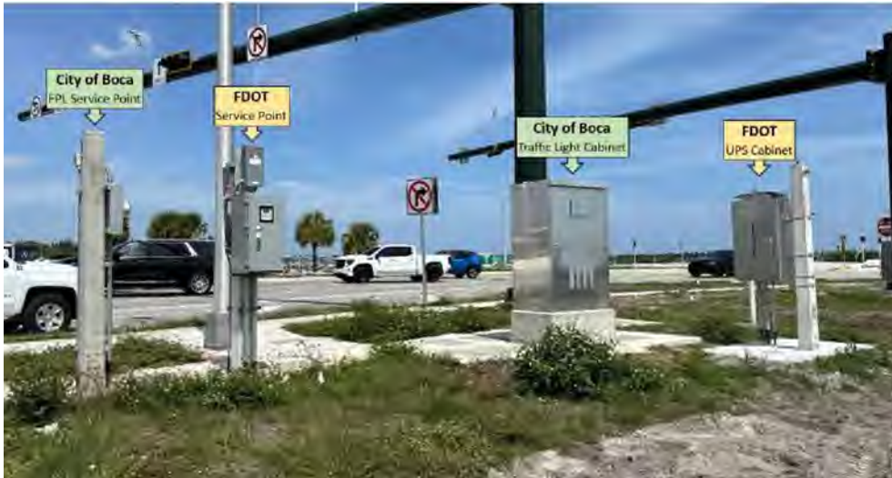
Figure 9: Cabinets at East and West Intersections
