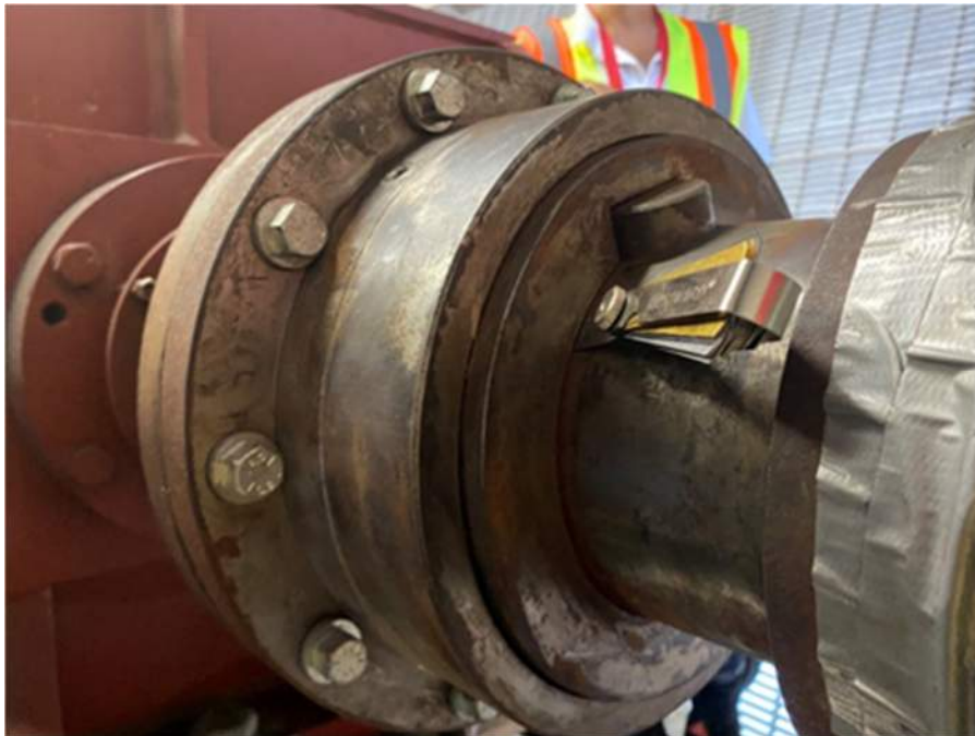
Photo 6: Clearance between the cracked hub and shaft, typical
