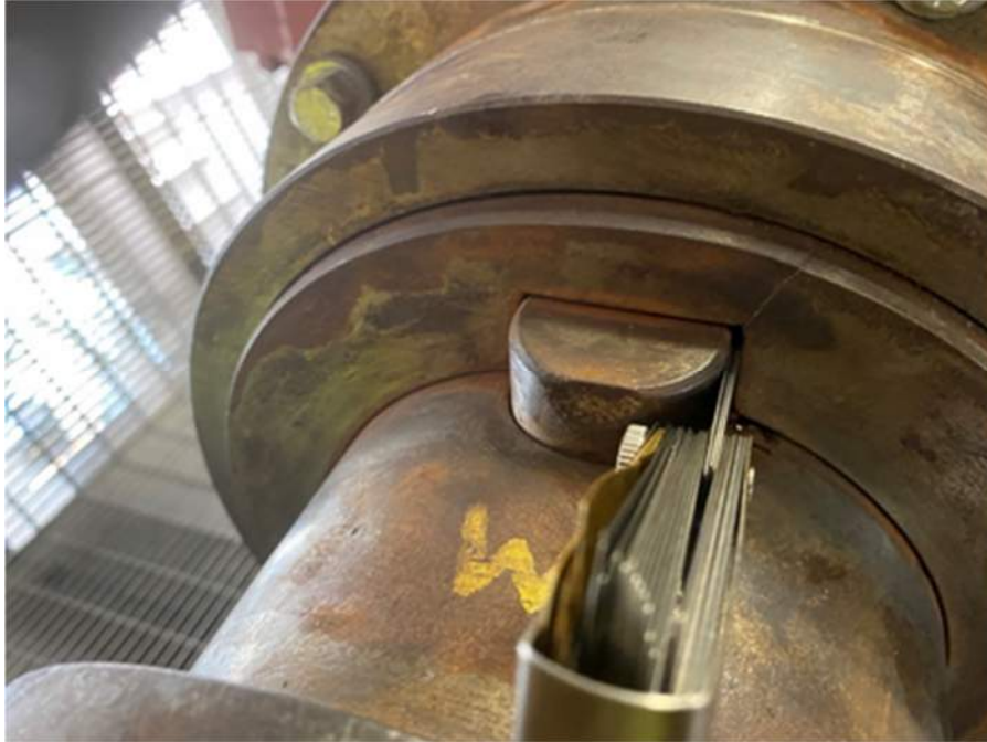
Photo 1: Side clearance between pinion hub key and keyway, typ. Note thru crack of hub
