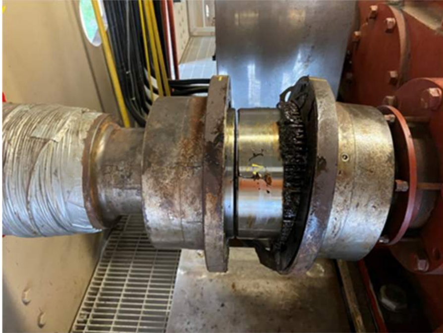
Photo 5: East coupling (bridge open position), note "small" gap between hubs
