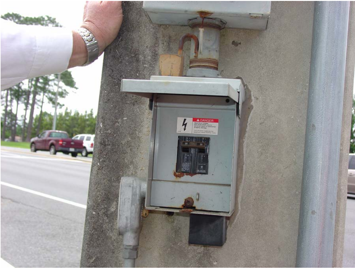
30 Amp Service at Apalachee Parkway and Executive Center Drive
