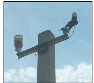
RWIS equipment installed in District Two to gather weather information.
