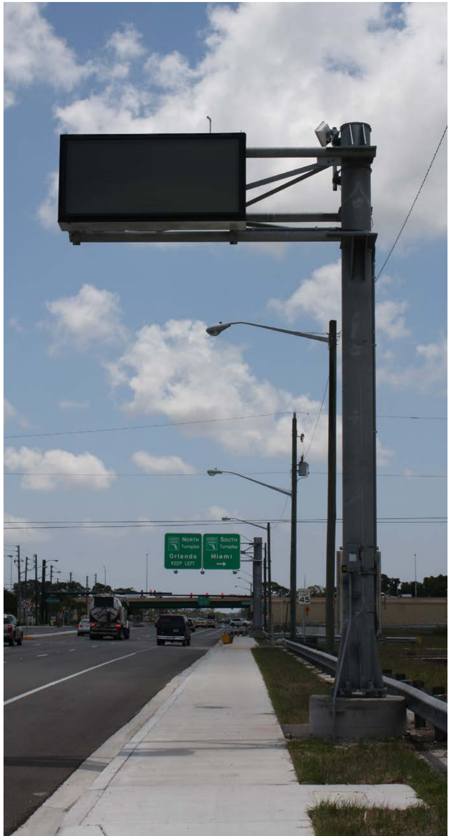
Older ADMS to be replaced.
