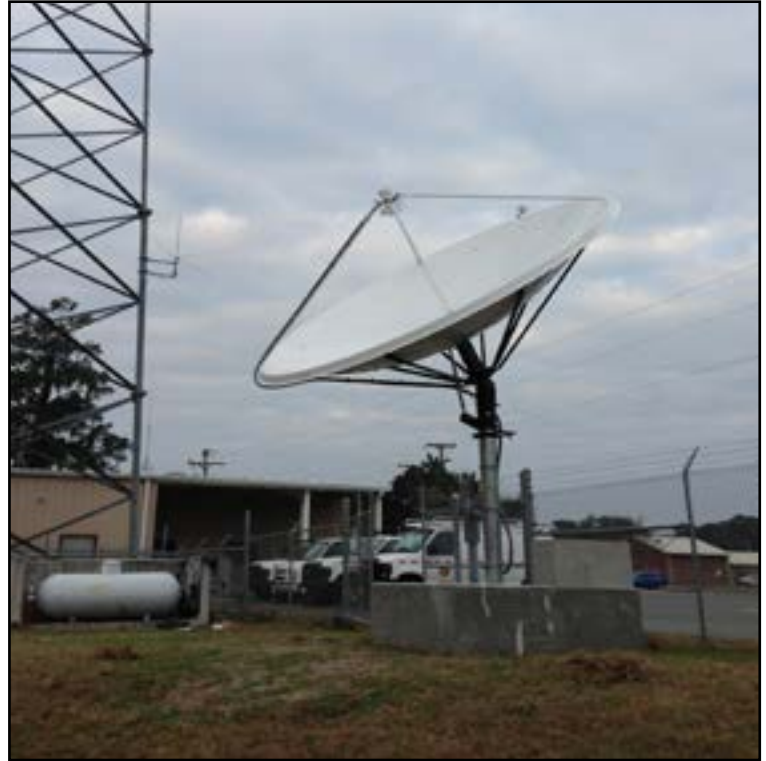
New FDOT satellite earth station at the District Two radio shop.
