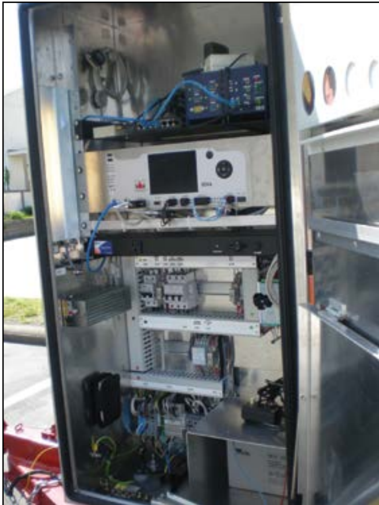
Typical cabinet at a signalized traffic intersection.
