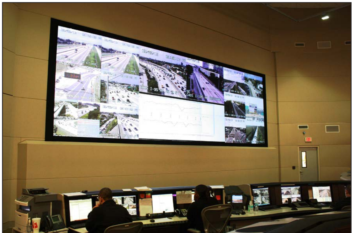
New video wall in District Six's SunGuide TMC.
