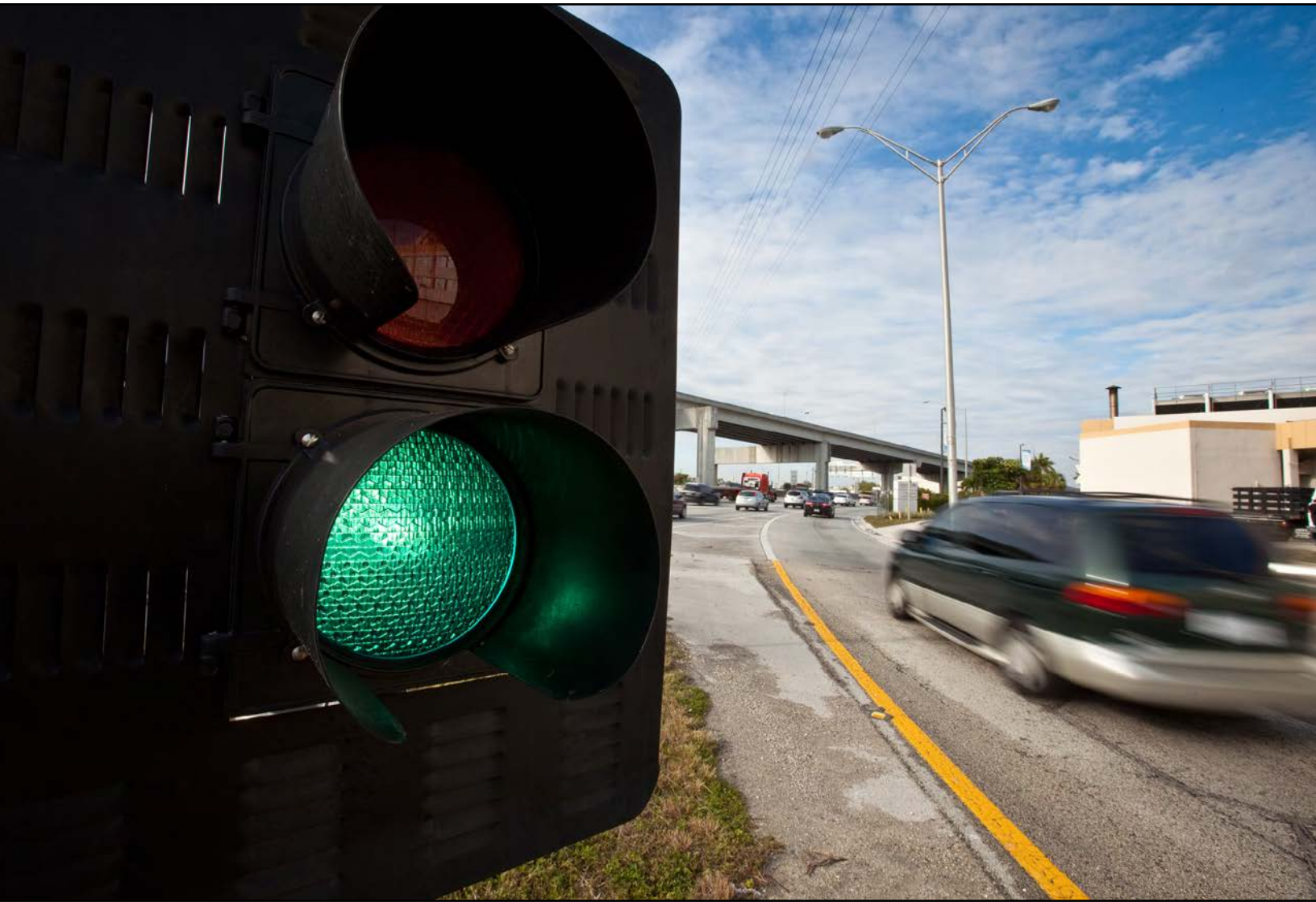
Ramp signaling in FDOT District Six.
