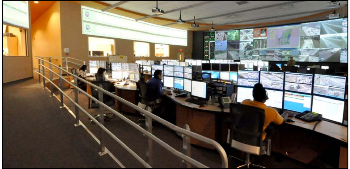
The Regional TMC now houses 22 workstations in the control room.
