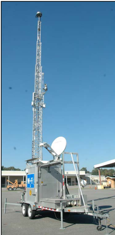
FDOT's mobile communications trailer.
