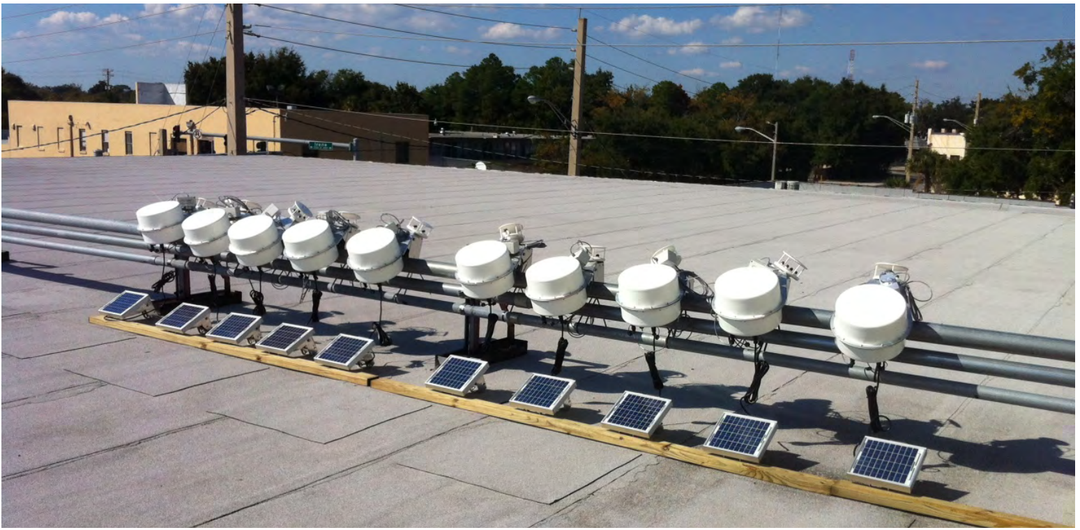
District Two roof-top calibration site.
