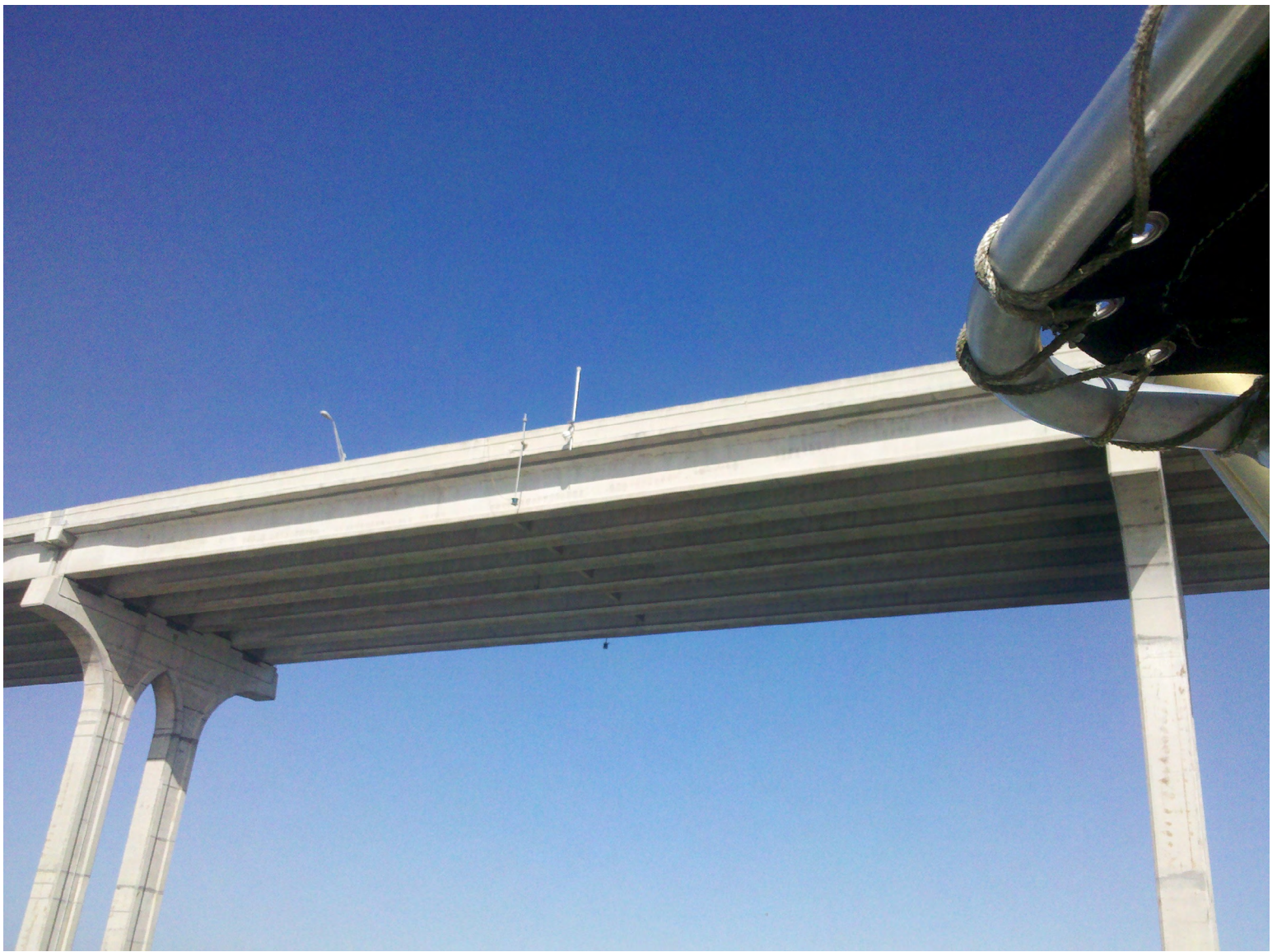
View of wind detection equipment on Vilano Bridge in Jacksonville
