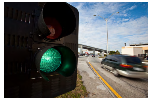
One of 22 ramp signals installed on I-95 turns green, signaling the vehicle to enter the highway.
