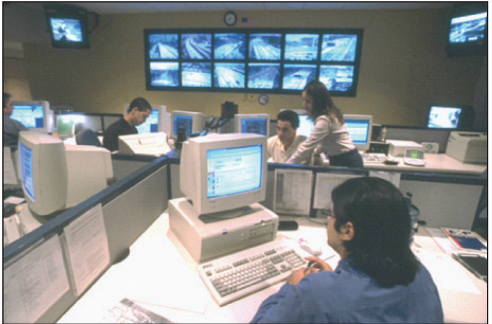
ITS Operations at the Interim Operations Center (pre-TMC).
