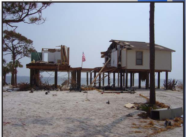
Damage from Hurricane Ivan, Escambia County.
