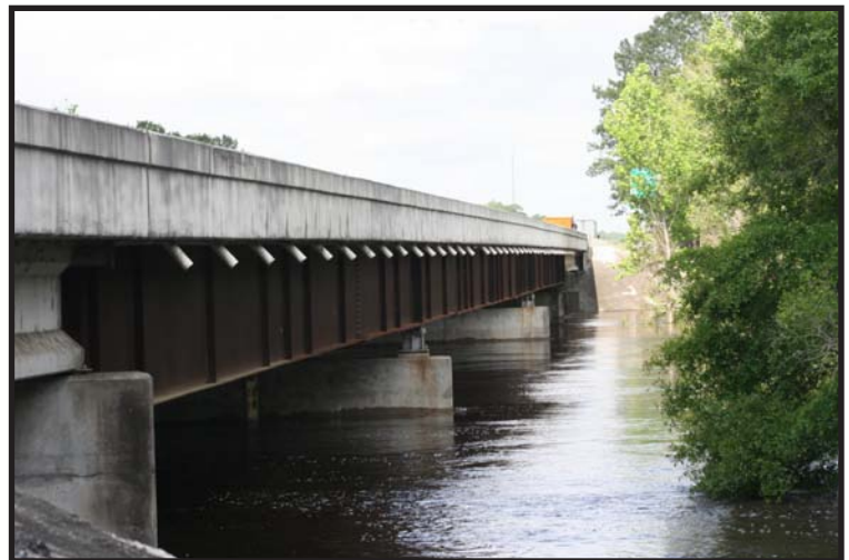
Suwannee River bridge west bound I-10, looking west under structure (provided by FDOT)
