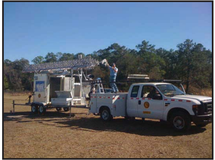
FDOT District 2 Radio Shop Personnel Deploying the Mobile WiFi Trailer.
