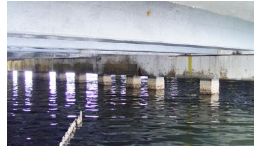
Before its replacement, this bridge developed severe corrosion concerns. The effectiveness of repairs made with FRP was shown in this project.
