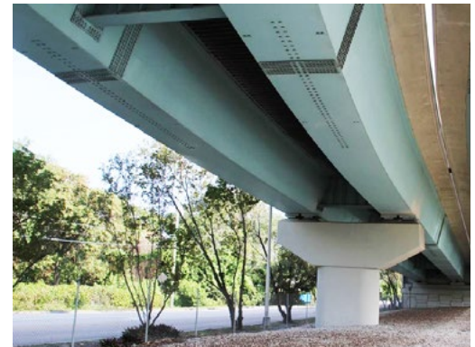
This view of one set of lanes on a Florida bridge shows the twin steel box girders and cross-braces.
