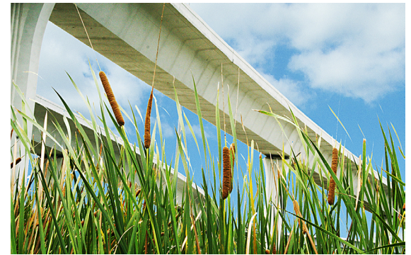
This Florida bridge depends on post-tensioning for its relative lightness and strength.
