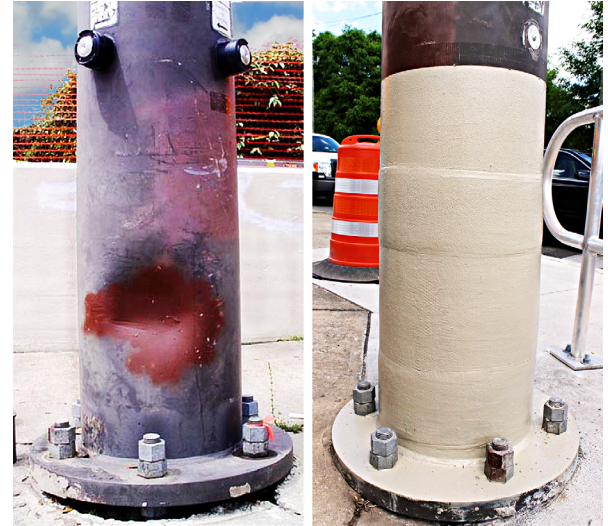
This utility pole (left) was damaged in a collision, but it was successfully repaired (right).
