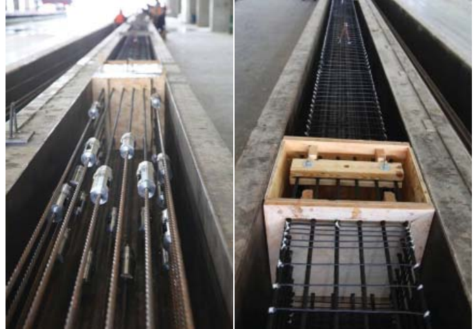
Left: a pile being constructed using steel prestressing strands. Right: a pile being constructed using CFCC prestressing strands.
