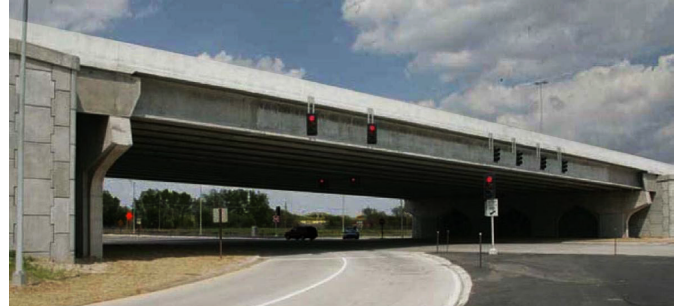
This bridge in Nebraska uses 207-ft spliced girders, similar to the type explored in this project.
