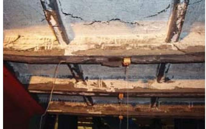
This post-test view of the underside of a UHPC-HSS bridge deck unit in an experimental setup shows the basic deck structure with primary and secondary ribs.
