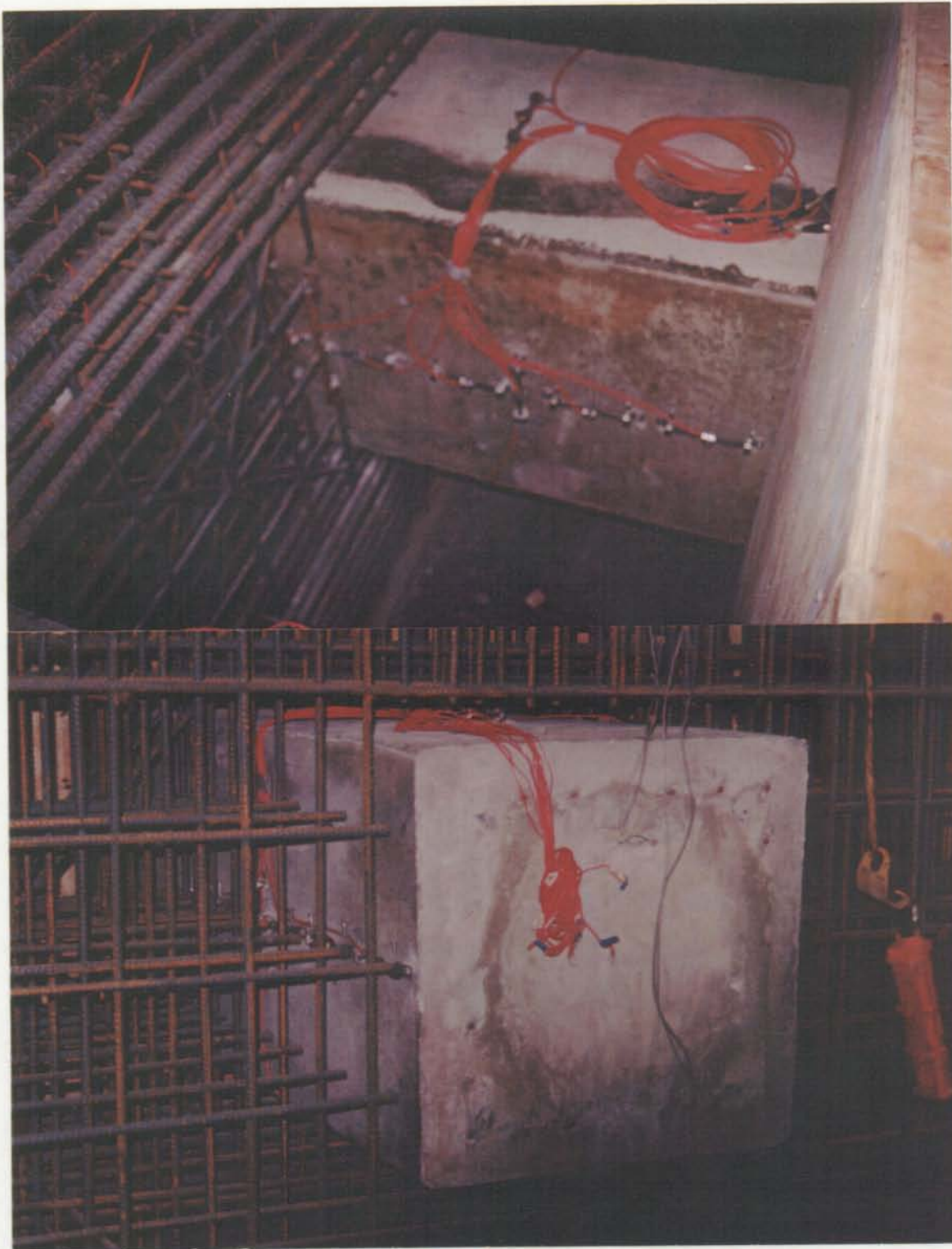
-Instrumentation of the 30" Square piles and the Pile Cap prior to Concrete Casting of the Pile Cap.
