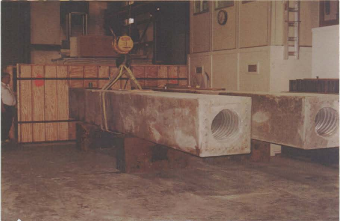
-Installation of the Modified Ends of the 30" PC Piles into the Pile Cap.
