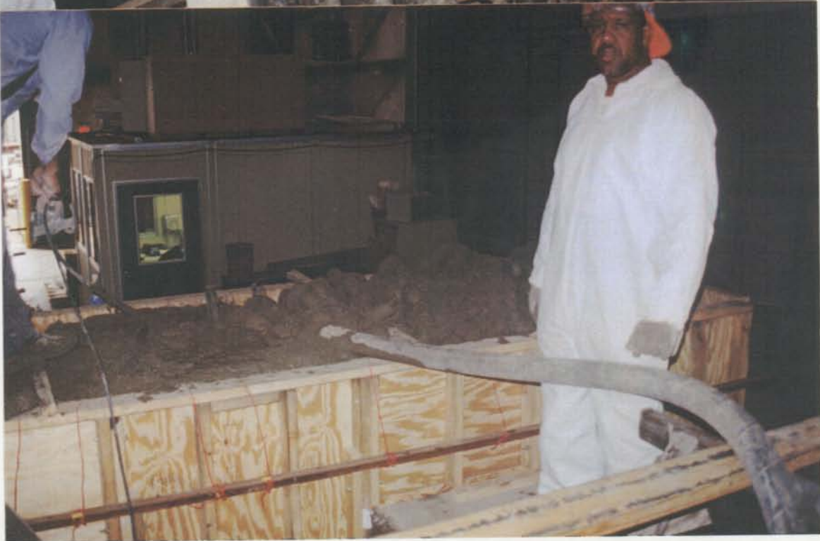
-Concrete Casting of the Pile Cap by using a Concrete Pump and an Interior Concrete Vibrator.
