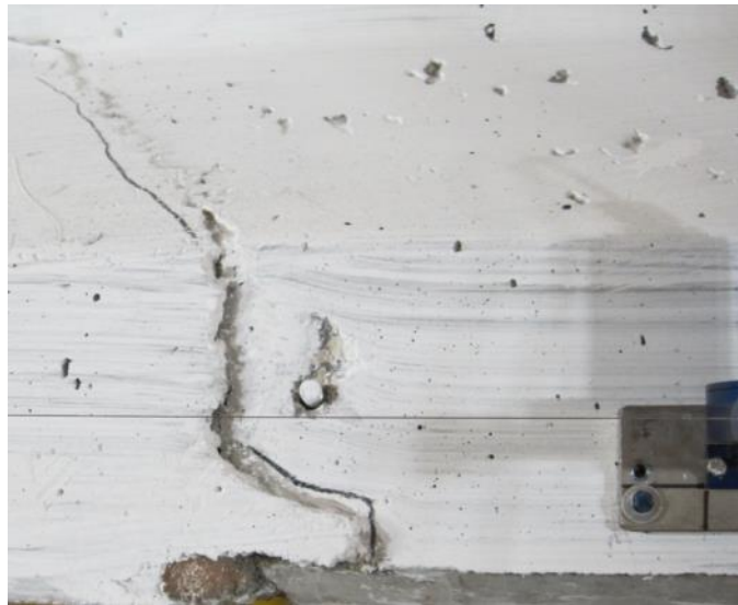
Figure 102-X1: Superficial cracks at overlap
