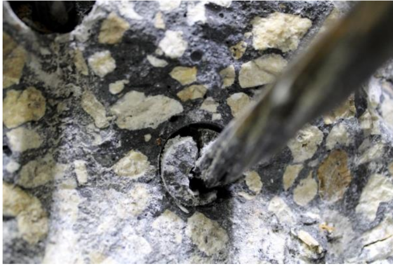
Figure 193–F2: Concrete intruding into unbonded length
