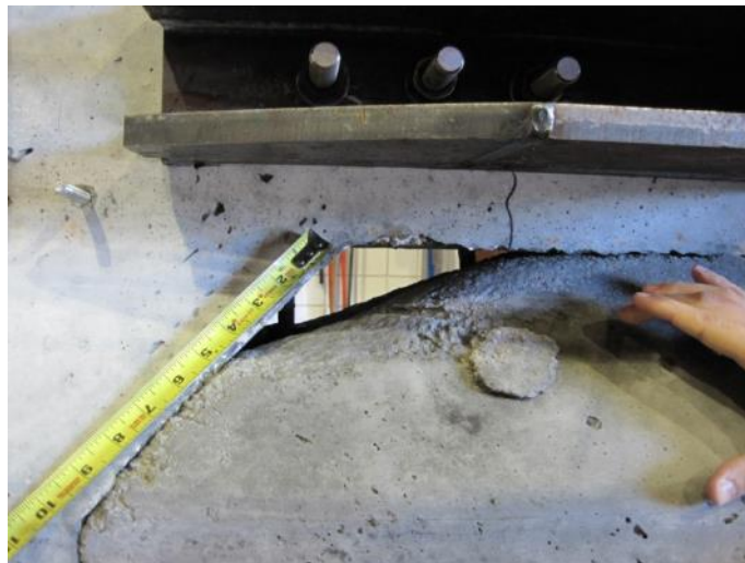
Figure 194–SB: Void at reentrant corner
