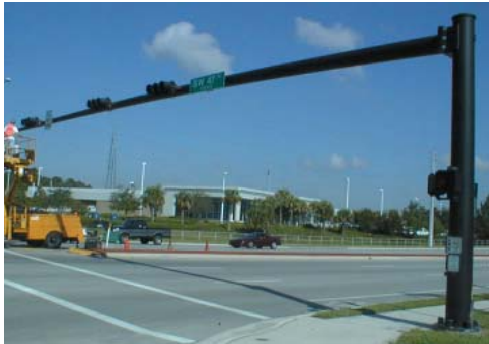
Figure 5.2 - Gainesville Long (70ft) Mast Arm
