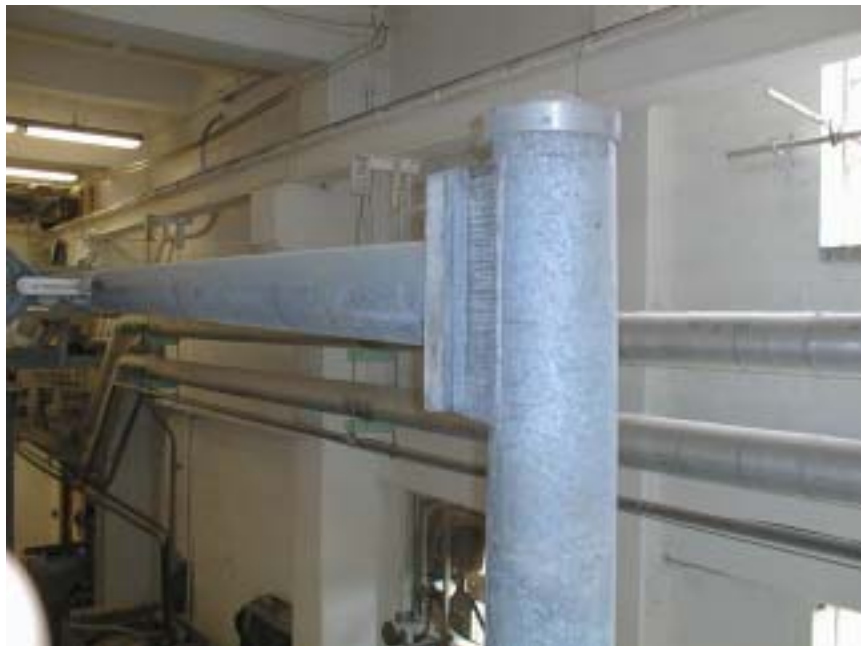
Figure 3.8 - Connection where Belleville Disc Springs and Neoprene Pads were installed
