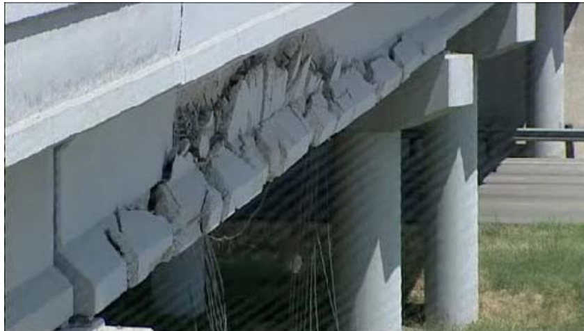
Figure 9.3. An example of damage from an over-height hit on a highway bridge
