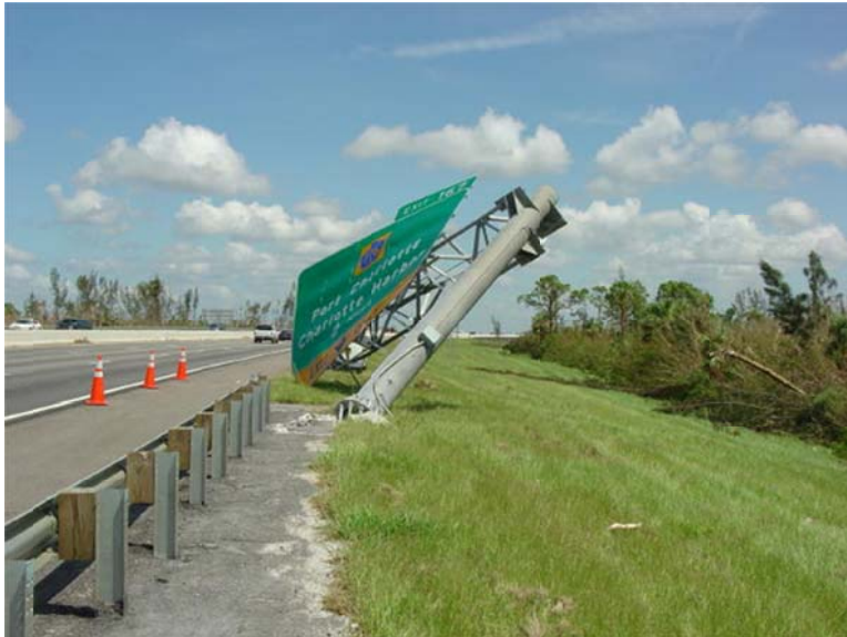
Figure 1-1. Failed cantilever sign structure. Photo courtesy of FDOT.
