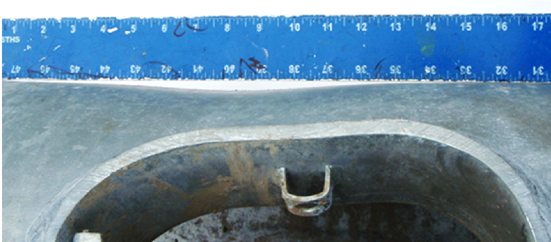
Figure 5-1. Pipe buckling near the access panel on the embedded pole. Photo courtesy of S. Dalton.
