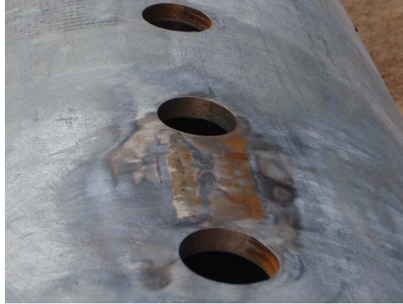
Figure 6-6. Rust on the surface of a pole and within the bolt holes. Photo courtesy of S. Dalton.
