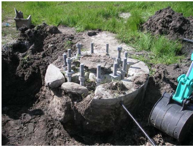
Figure 1-2. Failed concrete foundation of cantilever sign structure. Photo courtesy of FDOT.
