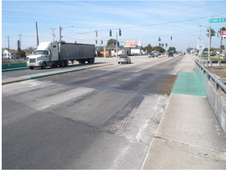
Figure 19 – Two northbound lanes showing truck traffic marks on the road surface.
