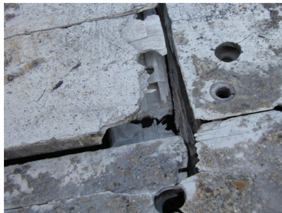
Figure 124 – Severe damage to top plates and webs
