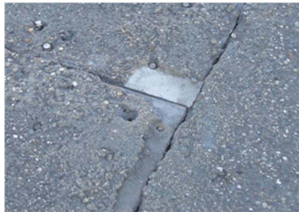
Figure 120 – Degradation at free edge
