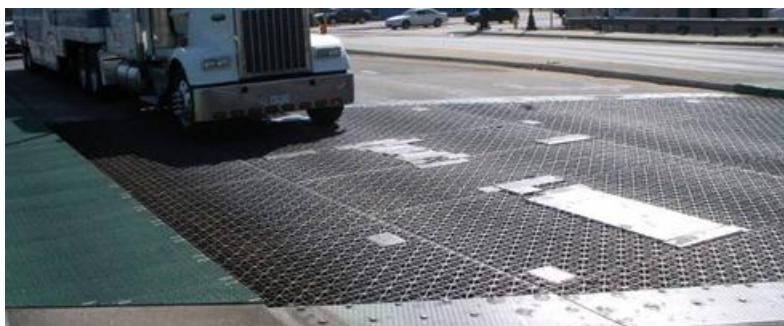
Figure 7 – Damaged and repaired existing steel grid deck
