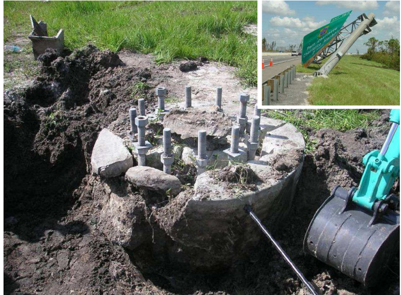
Partially excavated foundation showing concrete breakout that leads to collapse of the sign structure (inset, upper right).
