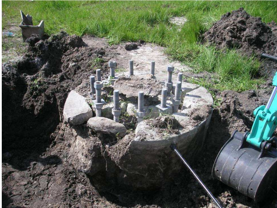
Figure 1-2. Failed foundation during post-failure excavation (1)
