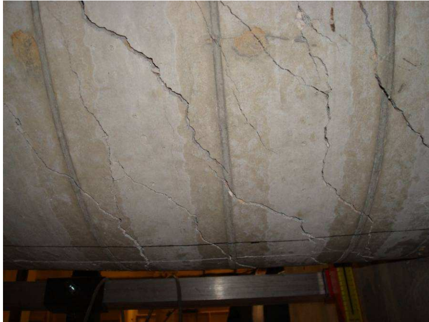
Figure 5-11. Widening of concrete breakout failure cracks in second test
