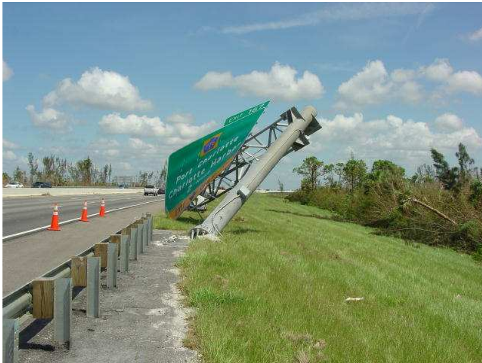
Figure 1-1. Failed cantilever sign structure (1)
