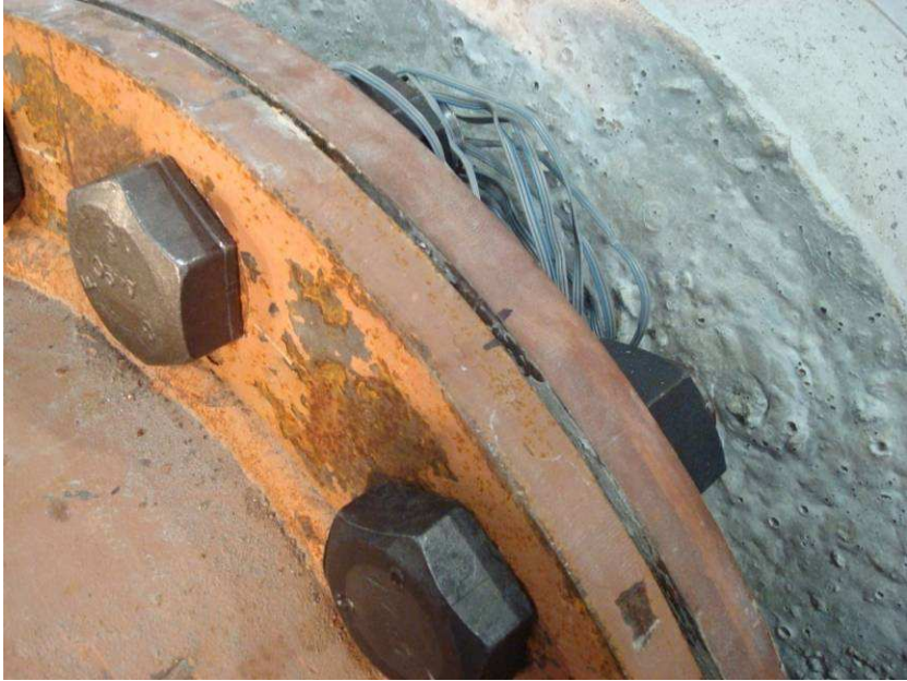
Figure 5-1. Lines drawn on base plate to show bolt slippage
