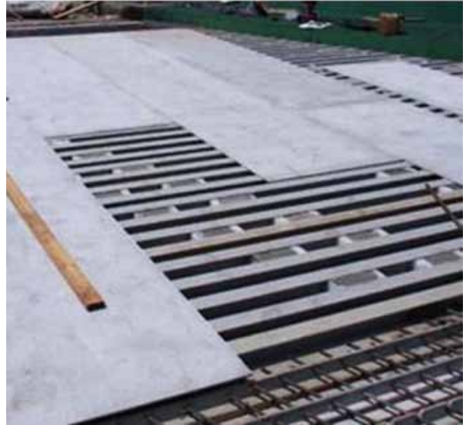
GFRP deck during installation shows the bottom layer, composed of interlocking I-beams. Top layer is being attached.
