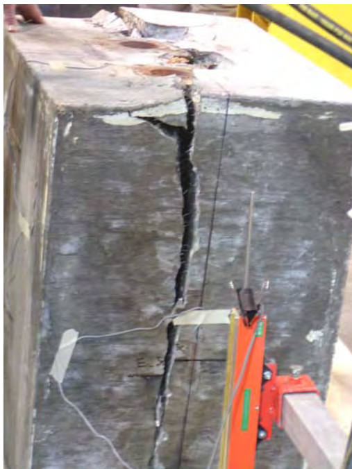
Figure 5-19: Punching Shear Failure of the Anchors in S1-2.
