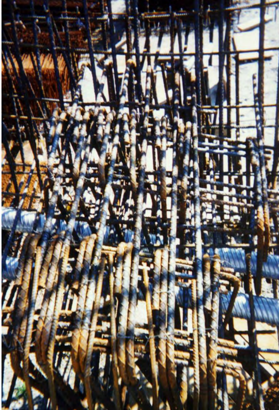
Figure 6-20: Close-up View of Steel Congestion in Post-Tensioning Anchorage Zone
