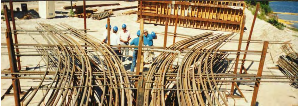
Figure 6-22: Roosevelt Bridge Pier Segment Reinforcing Steel with Fabrication Issues
