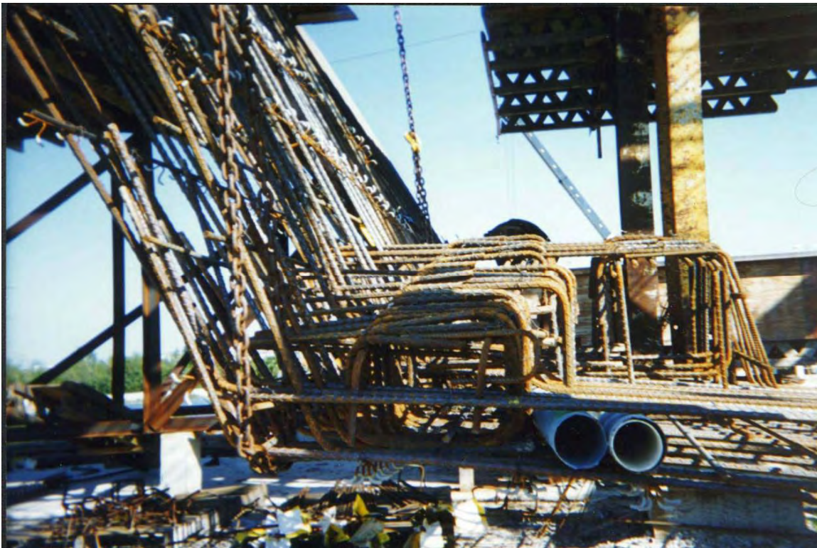
Figure 6-19: Steel Congestion in Post-Tensioning Anchorage Zone
