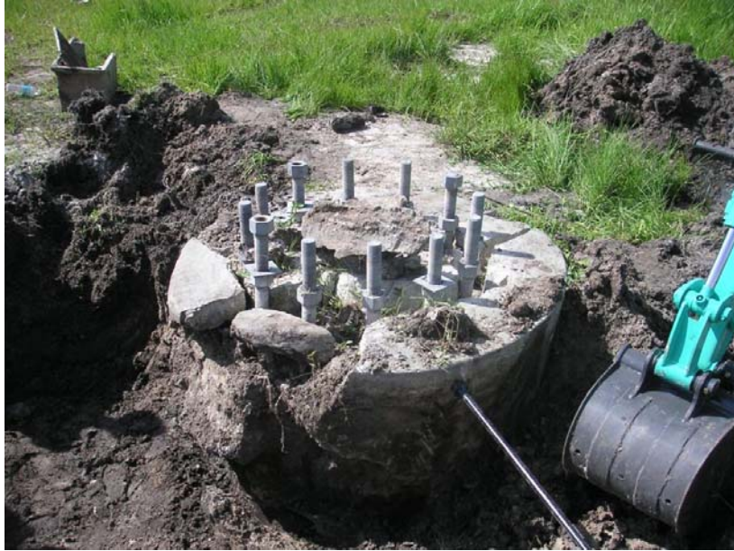
Figure 2-3. Failed foundation during post-failure excavation
