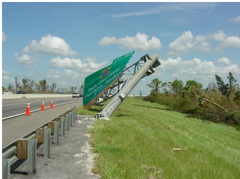
Figure 1-1. Failed cantilever sign structure
