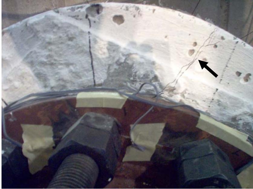
Figure 5-1. Initial cracks on face of shaft
