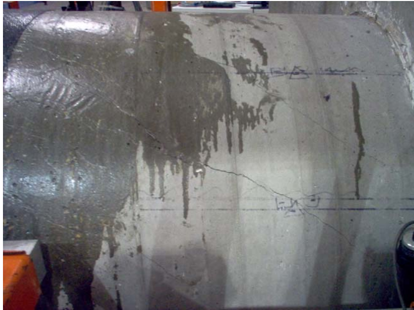
Figure 5-10. Shaft exhibiting characteristic torsion cracks from face to base of shaft
