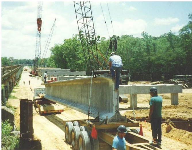
Figure 1.3 Transport of Florida bulb-tee girders to bridge construction site (State Road 20 Bridge over the Apalachicola River, Florida / Photo credit: Florida DOT)
