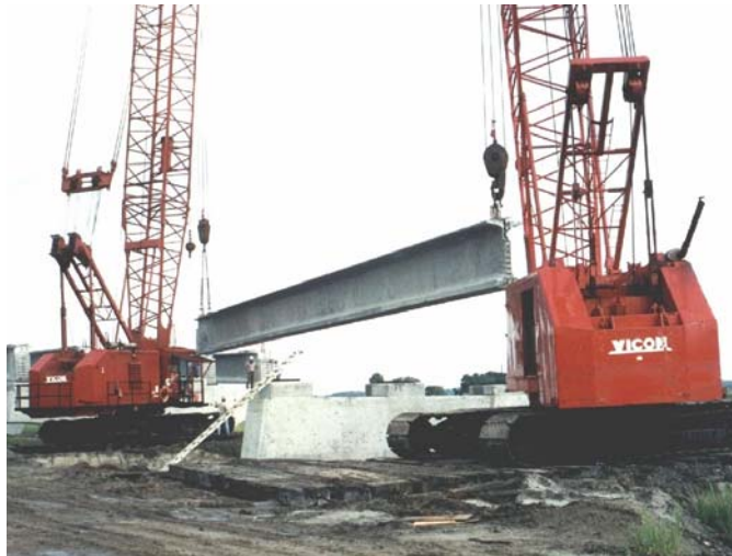
Figure 1.2 Lifting Florida bulb-tee girders for placement onto supports (Vilano Beach Bridge, Florida / Photo credit: Florida DOT)
