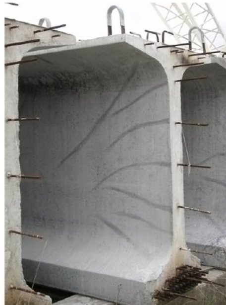
Preventing friction would reduce radial cracking like that shown in the I-beams above.
