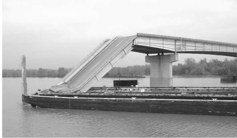
Figure 2.4 Collapse of an Interstate I-40 bridge in Oklahoma (2002) after being struck by a barge flotilla (Source: Oklahoma DOT)
