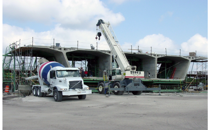
Construction of concrete bridge segments from the John Ringling Causeway, Sarasota, Fla.
