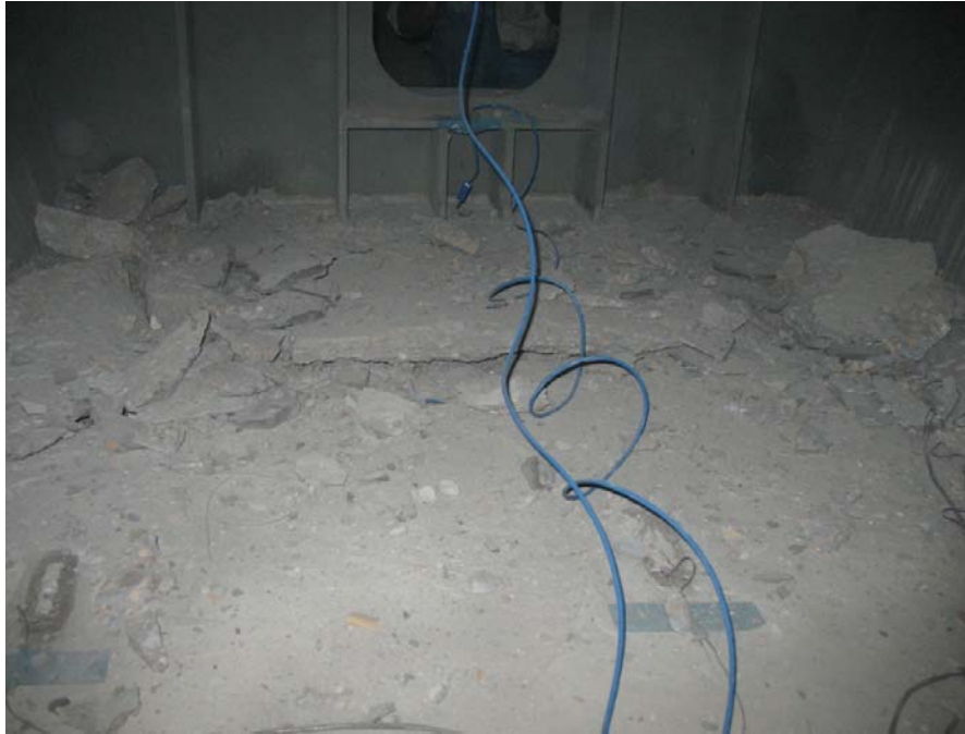
Figure 9.1 Bottom Slab Showing the Extent of Concrete Crushing
