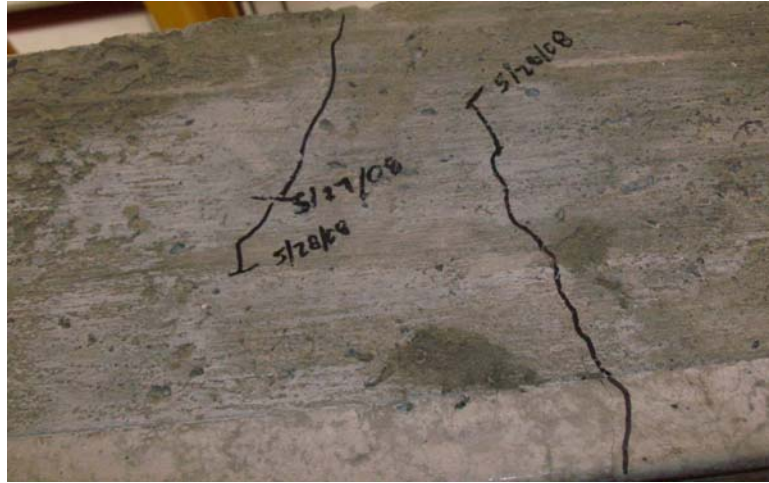
Figure 5.12 Structural Cracks at Intermediate Support on Hold Down Side
