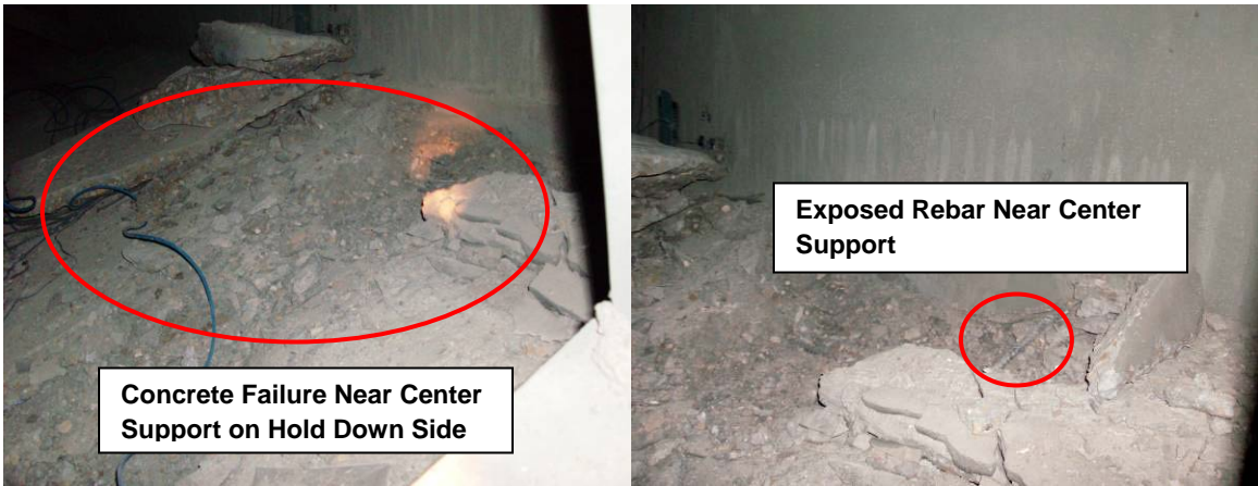
Figure 7.4 Failed Bottom Concrete Slab on Hold Down Side
