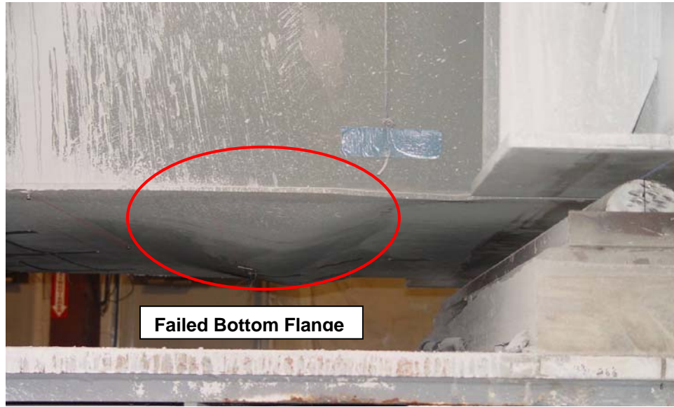
Figure 7.1 Failed Bottom Flange on Hold Down Side
