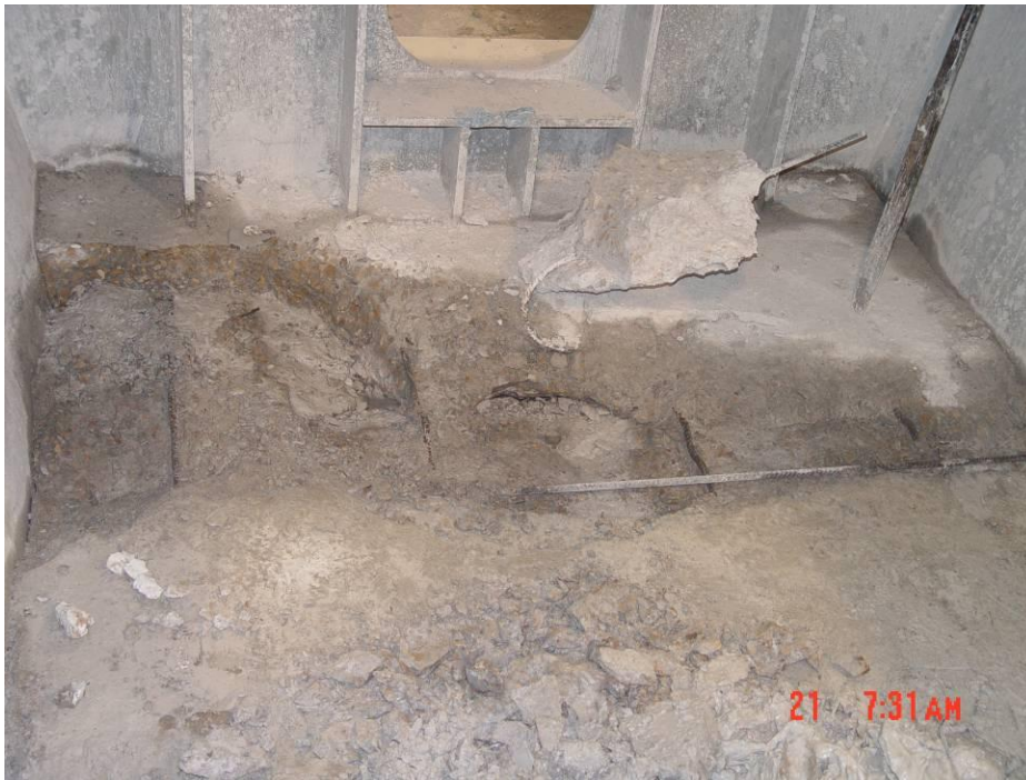
Figure 7: Concrete Failure (Removal of Loose Pieces)
