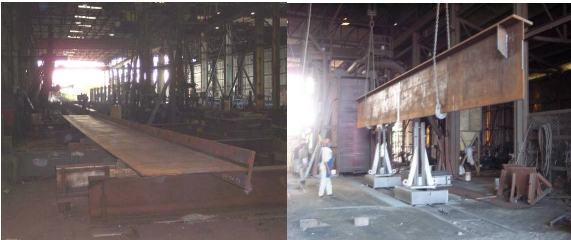
Figure 3.4 SAC Welding of Top Flange/ Web and View of Assembly Prior to Shot Blasting
