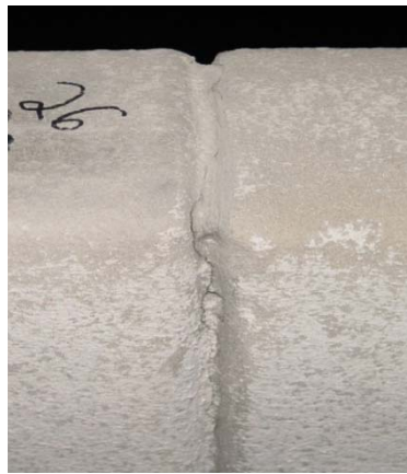
Figure 13: Tension Cracks within Control Joint.
