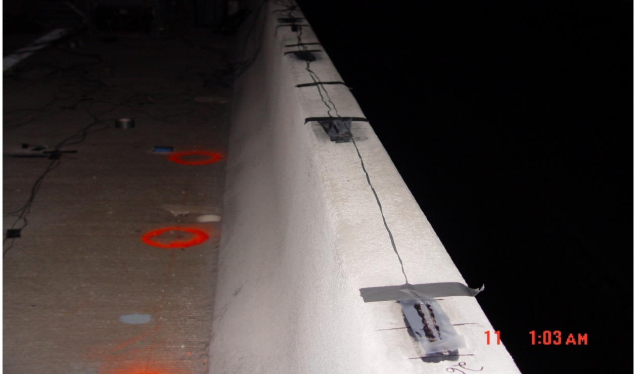
Figure 36: Longitudinal Barrier Strain Gages.
