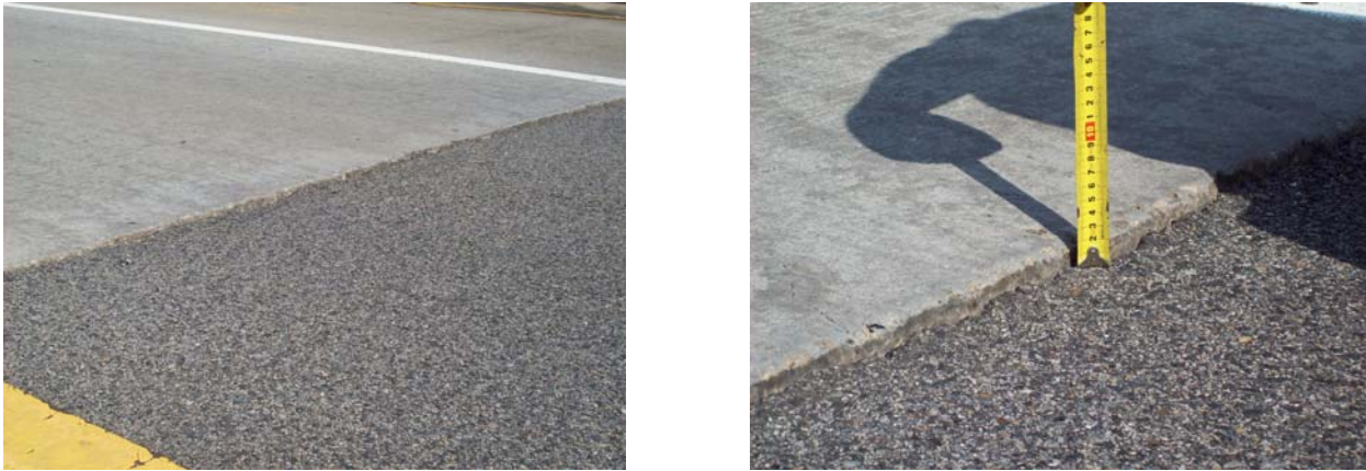
Figure 3.3. Bridge approach depression and a protrusion on the boundary of asphalt pavement and concrete slab
