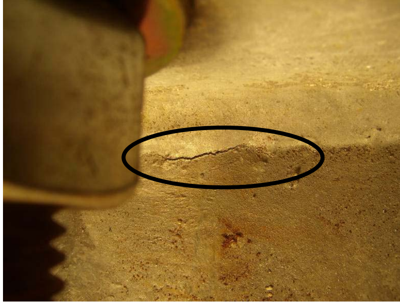
Figure 7. Cracking in the Toe Weld
