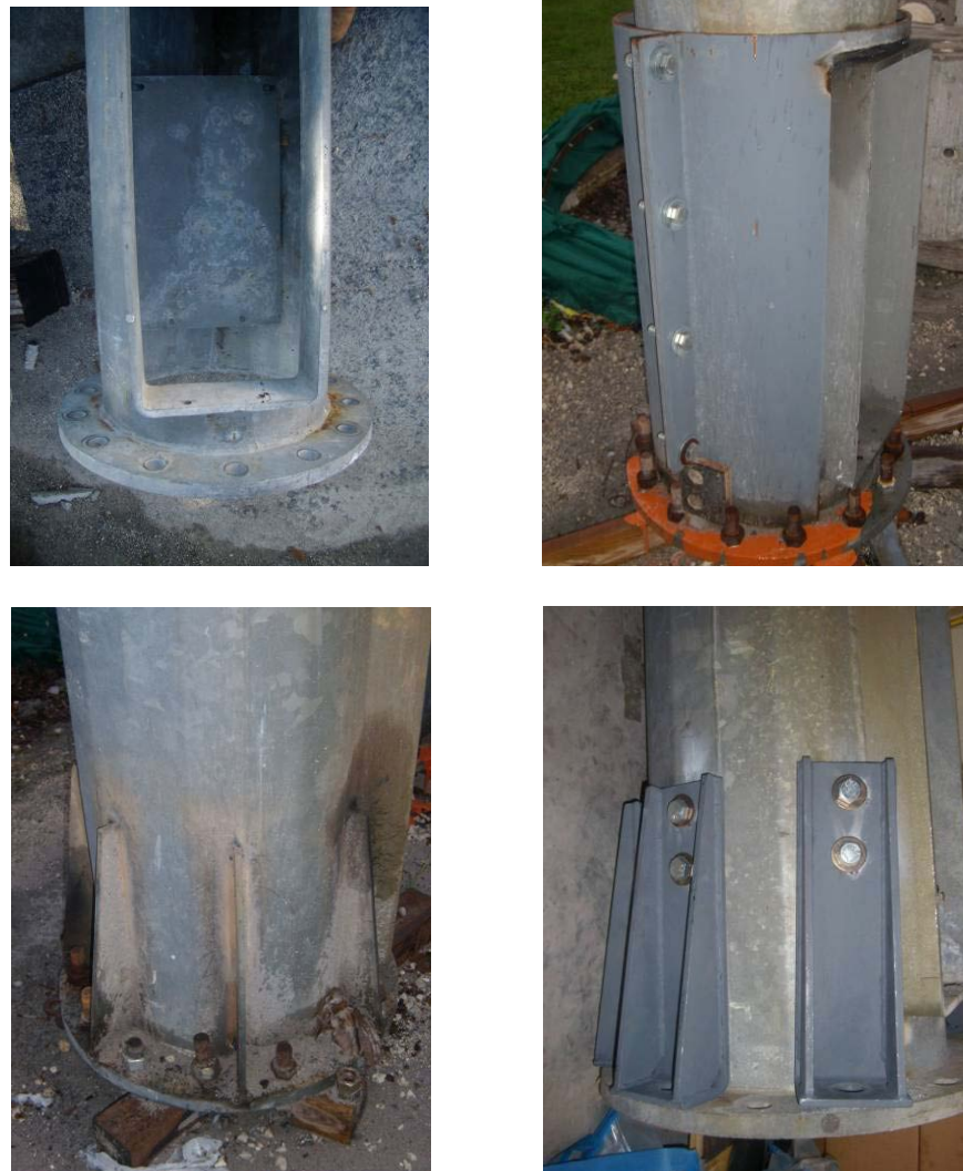
Figure 3. Installed Specimens (Clockwise from top left: Reweld, Steel Jacket, Welded Plate, Bolted Plate)
