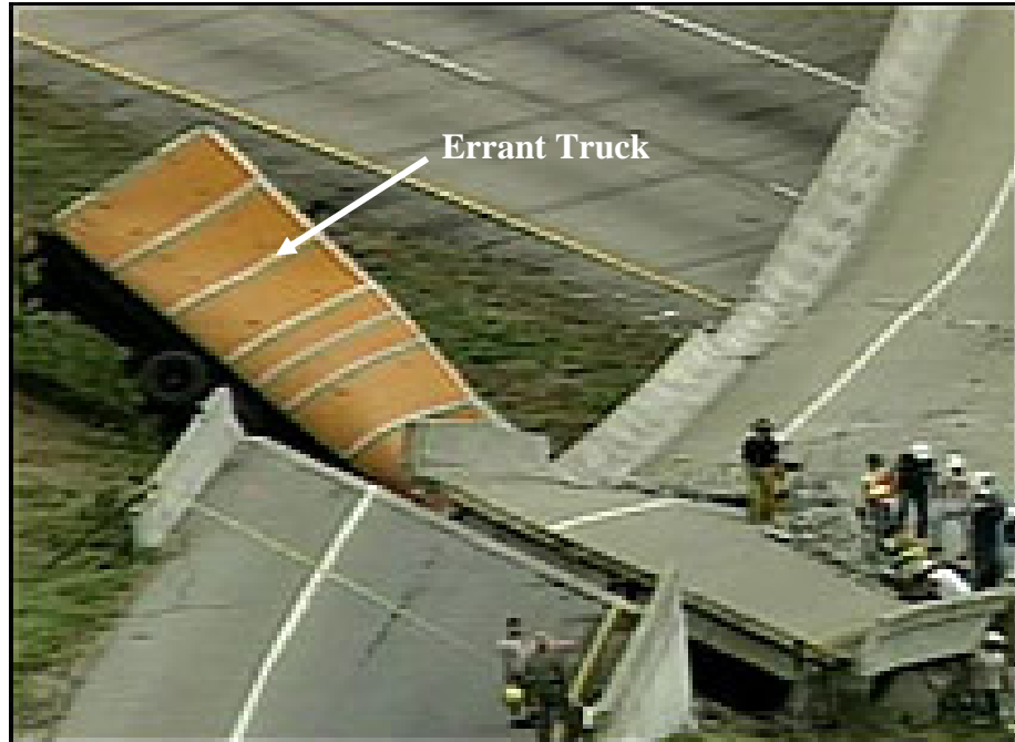
Figure 1-1: Collapse of I-45 bridge (near Dallas, TX) after being struck by tractor trailer (Sept. 2002).
