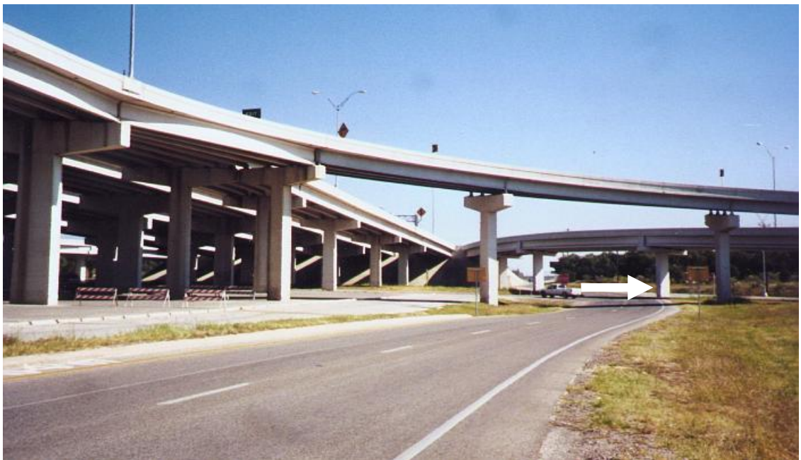
Figure 1-4: Unprotected bridge piers. The marked column is especially vulnerable because it is at the end adjacent to a curve in the highway.
