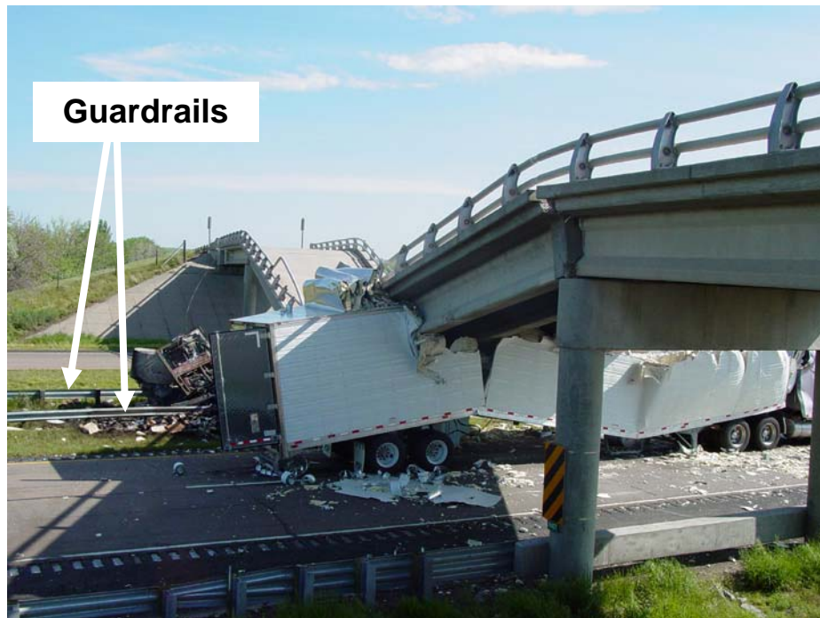
Figure 1-2: Collapse of I-80 bridge (near Big Springs, Nebraska) after being struck by tractor trailer (May 2003). Photo: courtesy of NDOR.
