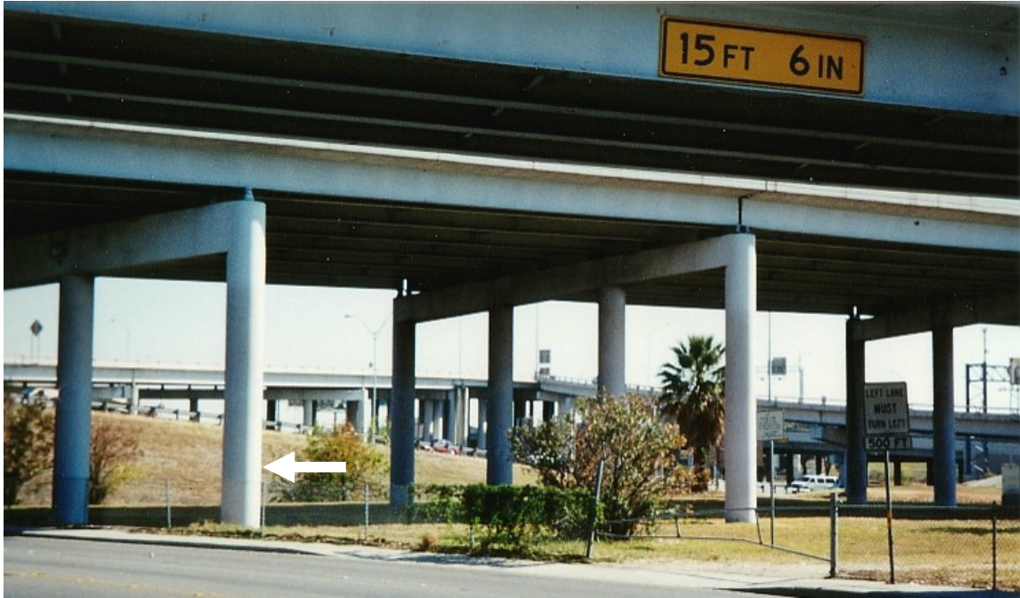
Figure 1-5: Vulnerable bridge piers. The marked column is quite small and can be seriously damaged in a head-on collision.
