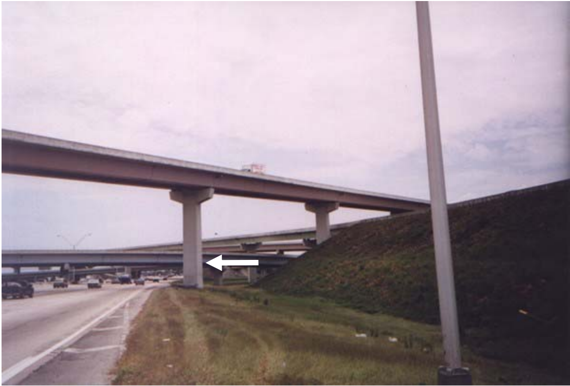
Figure 1-3: Vulnerable bridge pier. The column is protected by a barrier, which appears to be rather inadequate to protect against head-on impact by a heavy truck.
