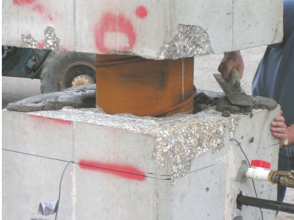
Figure 4-7 Steel bolts greased and inserted to support HSS pipe, annulus grout globe valve was attached with epoxy, and mating surface grout was applied.
