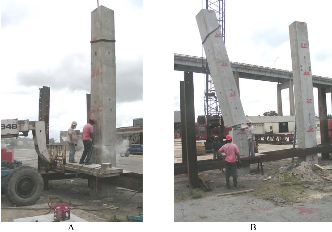
Figure 4-3 Pile cutoff to expose void. A) Concrete pile is cut with diamond blade circular saw; B) metal liner of pile void is cut with an oxyacetylene torch.
