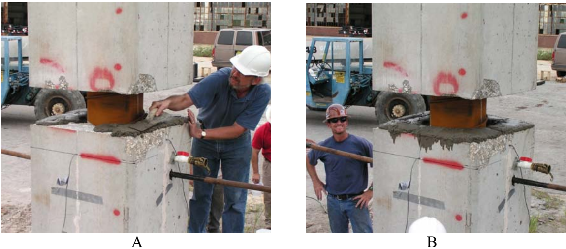
Figure 2-6 The Set 45 mating surface grout. A) Apply mating surface grout, B) ready to lower the top pile into position.
