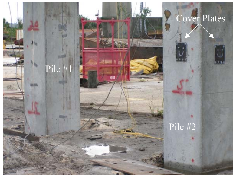
Figure B-4 Bottom set of instruments, with steel cover plates attached on Pile #2; Pile #1 driven to cutoff elevation with tip at -14 feet.
