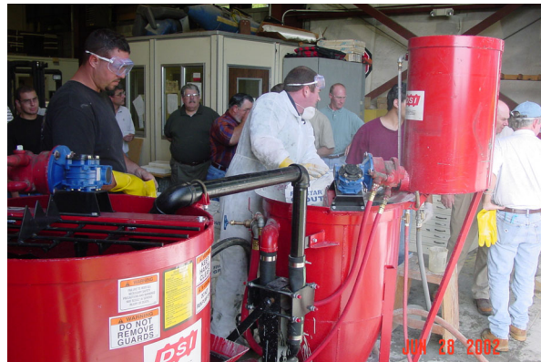
Figure 1 - Colloidal Mixer and pump used to mix and inject grout for Wick-Induced Bleed Tests. Photo shows DSI personnel adding bagged grout to mixer during mixing operation.
