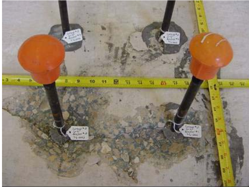
Figure E-11 Typical grout/concrete failure of quadruple fastener anchor group with anchor spacing of 9 inches
