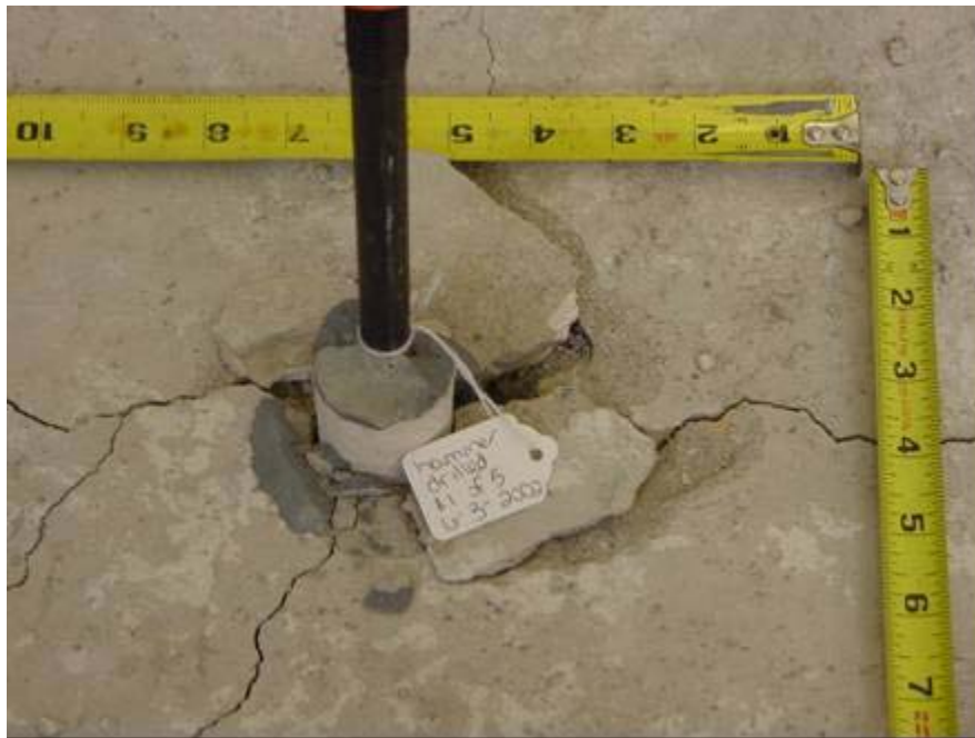
Figure E-4 Typical grout/concrete bond failure of single hammer-drilled anchor with grout plug
