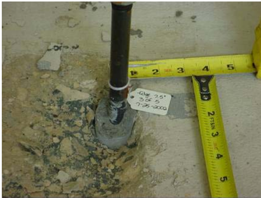
Figure E-8 Typical grout/concrete bond failure of single core-drilled anchor installed 7.5 inches from one edge with grout plug
