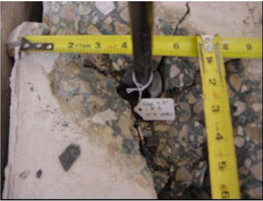
Figure E-6 Typical grout/concrete bond failure of single core-drilled anchor installed 4.5 inches from one edge with grout plug and diagonal cracking of surrounding concrete
