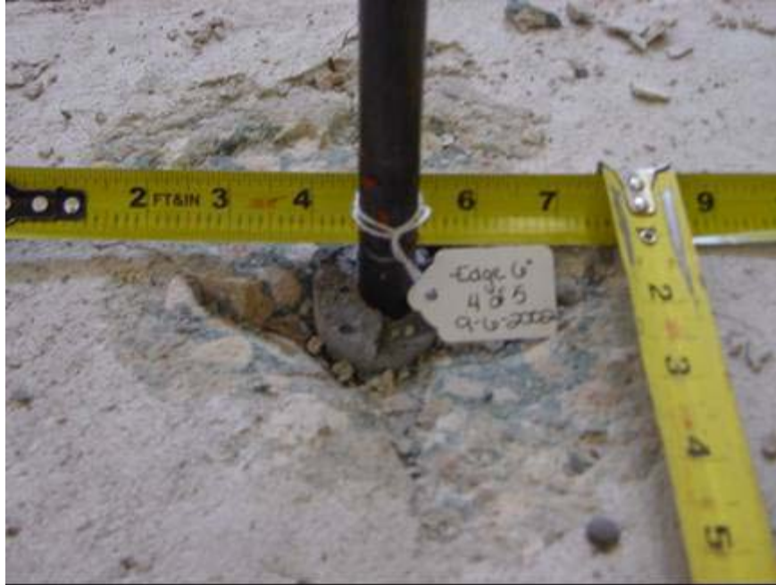
Figure E-7 Typical grout/concrete bond failure of single core-drilled anchor installed 6.0 inches from one edge with grout plug
