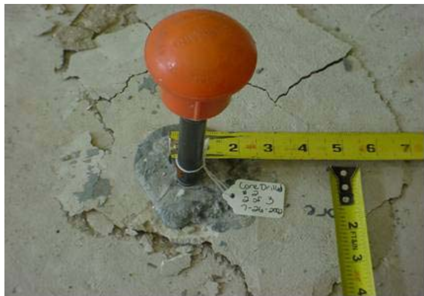
Figure E-2 Typical grout/concrete bond failure of single anchor with secondary shallow concrete cone
