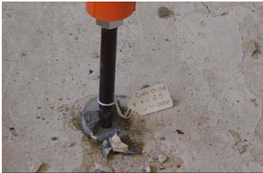
Figure E-1 Typical grout/concrete bond failure of single core-drilled anchor with grout plug
