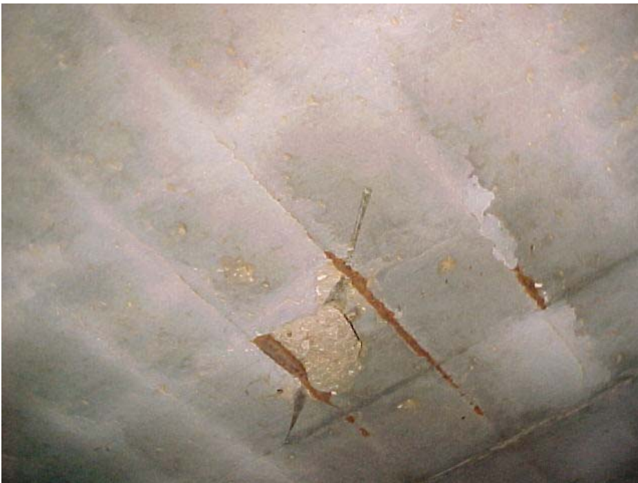
Figure 3.5: Exposed and Corroded Reinforcing Steel
