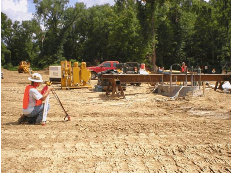
Figure 4-120 Natchez: Field survey during post grouting (quality assurance testing of post grouting).
