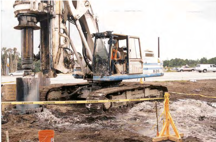
Figure 4-7 PGA Blvd: Clean-out of bottom to ensure cleanliness of bottom prior to cage placement.
