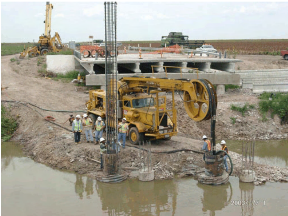
Figure 4-145 FM 507: Reinforcement cage placement in west shaft and de-sanding of east shaft.
