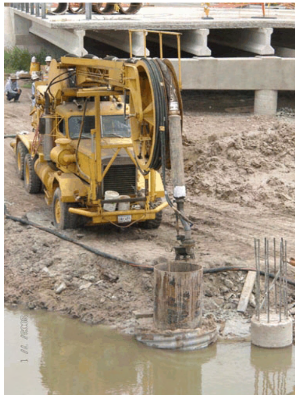
Figure 4-143 FM 507: Submersible de-sanding pump.
