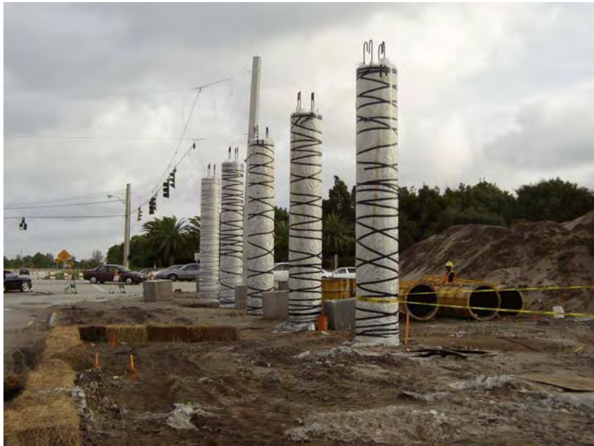
Figure 4-32 PGA Blvd: End bent 4 columns.
