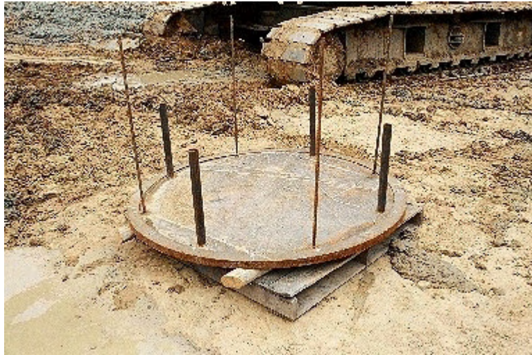
Figure 4-115 Natchez: 60 inch diameter grout plate.
