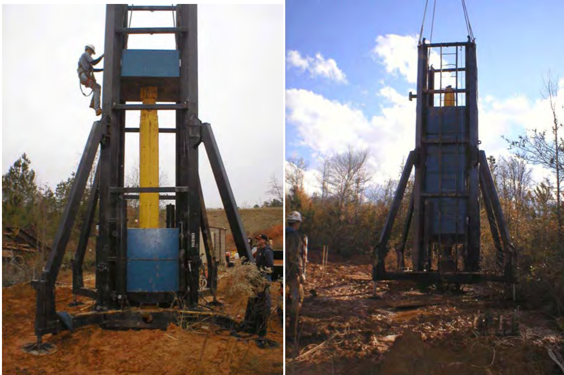
Figure 4-68 NGES Auburn: USF & FHWA's 4 MN Statnamic hydraulic catching device.
