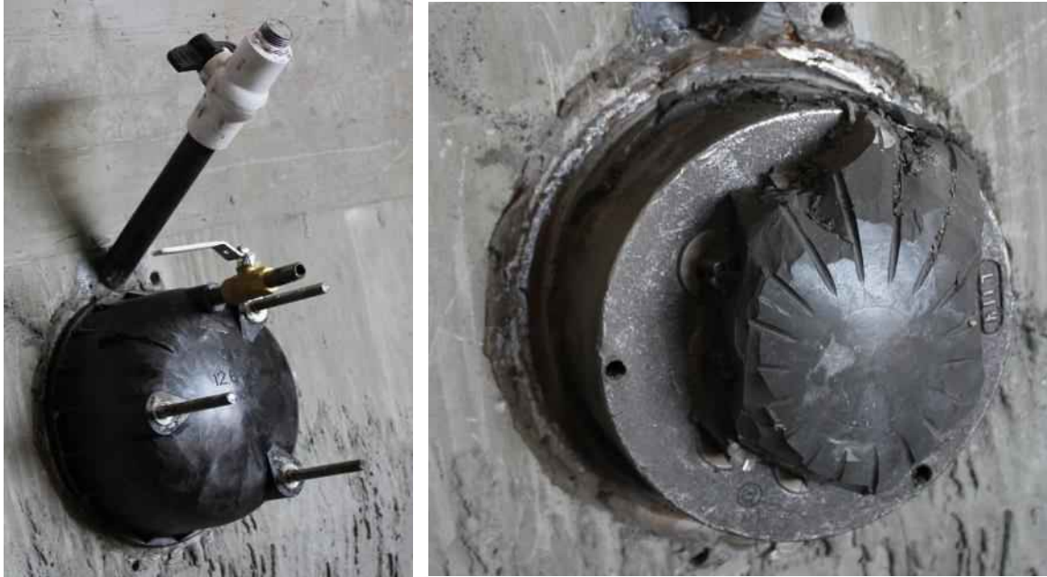
Figure 6-12 IGS inlet (live end) prior to and after cap removal (damaged)
