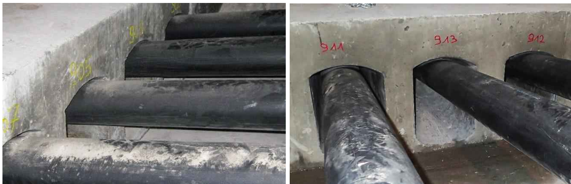
Figure 4-16 Tendons with point of contact located inside deviator. Note small gap between duct and concrete at tendon exit from deviator.
