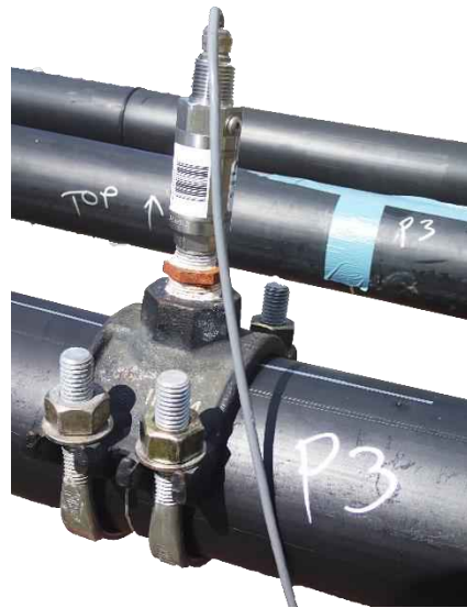
Figure 6-4 Typical transducer installed on the tendon
