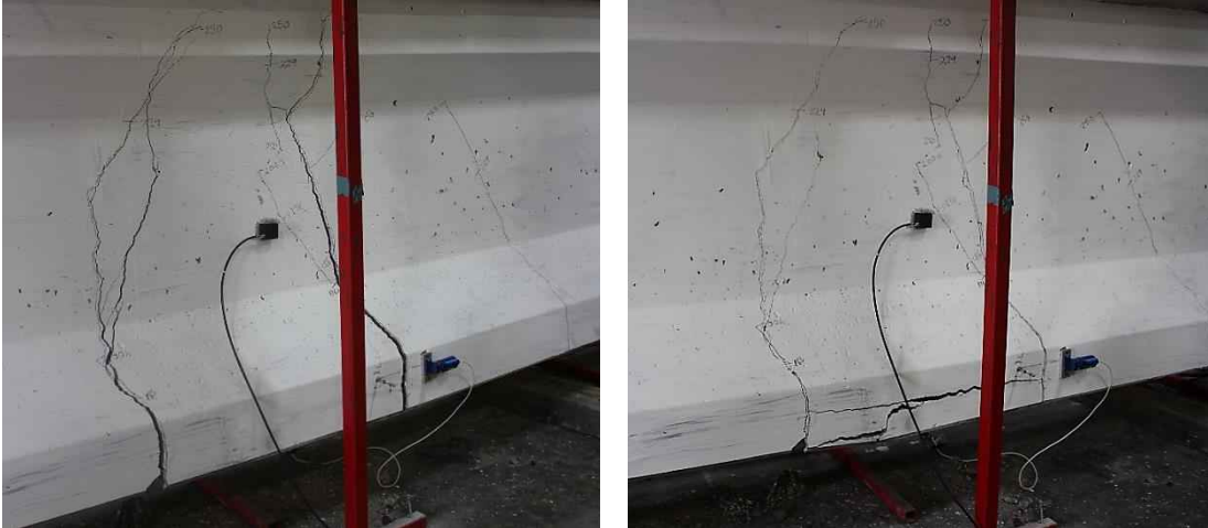
Figure 10-7 Cracking (a) after strand rupture, load held at 240 kip and (b) after load removed
