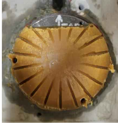
Figure 6-16 Inlet (live end) after cap removal of IWS
