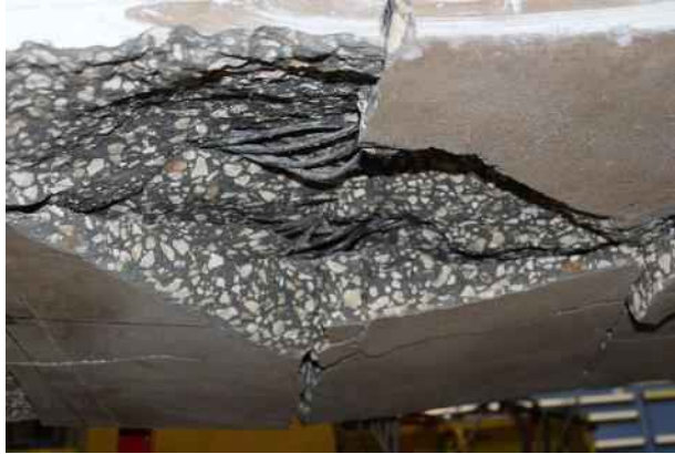
Figure 10-14 IWC: ruptured bonded strands
