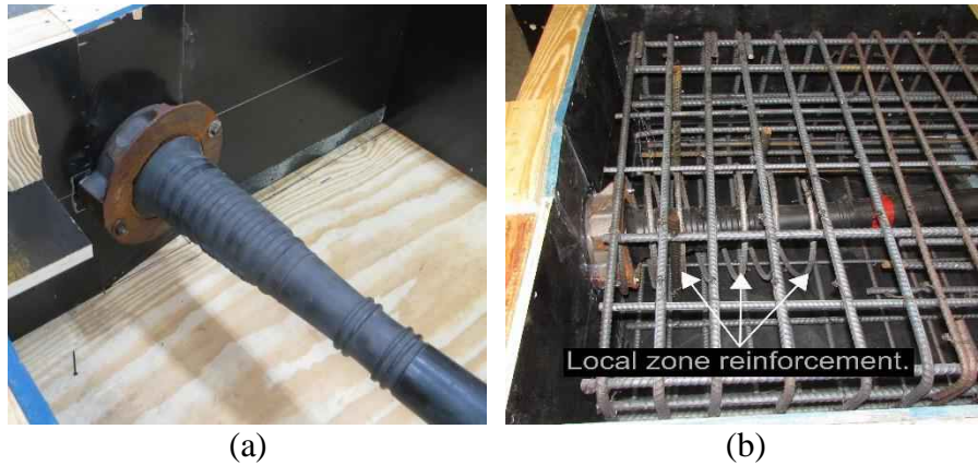
Figure 4-19 Anchorage system (a) without local zone reinforcement (b) with local zone reinforcement
