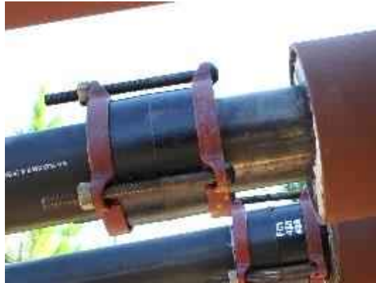
Figure 5-11 HDPE duct connected to the anchor block at the east end
