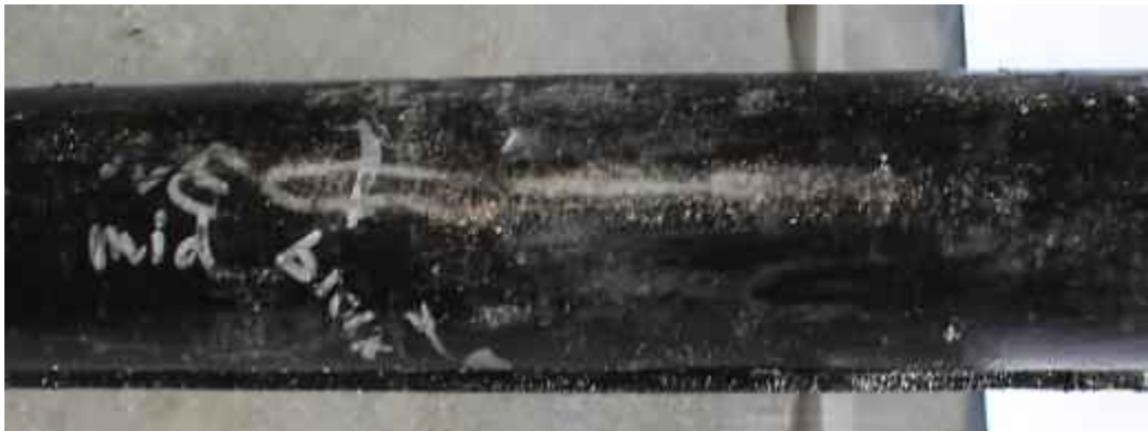
Figure 11-21 EWC: exterior surface of duct at NE diabolo
