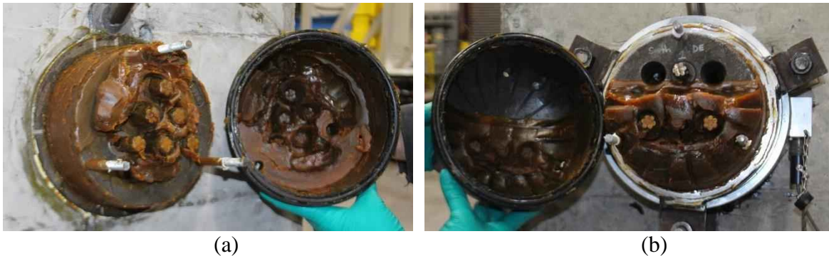
Figure 6-45 F1 anchor after injection at (a) live end and (b) dead end
