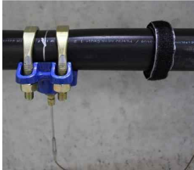
Figure 5-10 Probe (left) and surface strap (right) thermocouples
