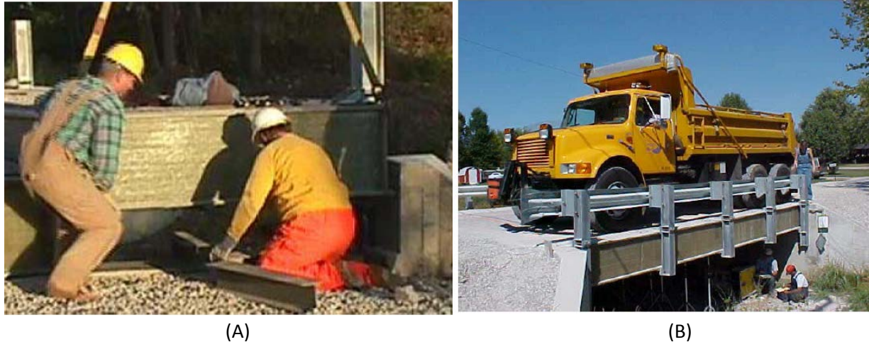
Figure 17. St. Francis Street bridge, St. James, MO, November 2000 [42]. (A) Installation and (B) load testing.
