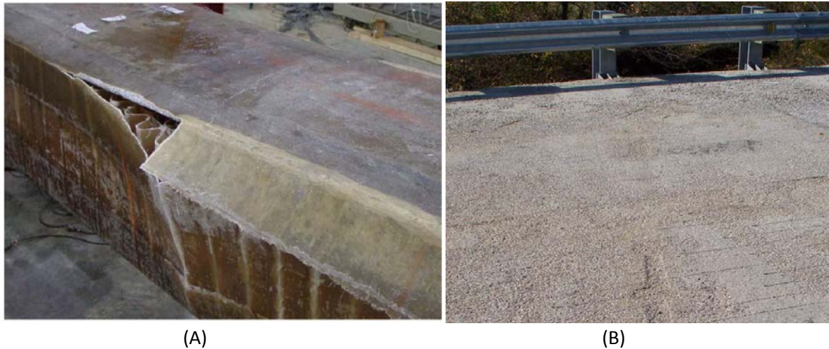
Figure 19. Flat-slab FRP honeycomb bridge for Huron County, Ohio [44]. (A) Failure mode of sample from laboratory experiment and (B) polymer concrete wearing surface showing degradation after ~3 years of service.
