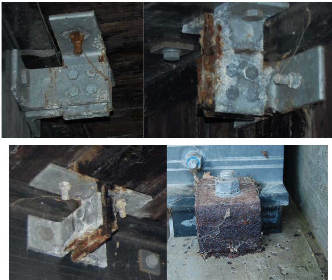
Figure 123. Corrosion of metallic components on pultruded FRP girder bridge (Dickey Creek bridge, Route 601, Sugar Grove, VA) Photos taken December 26, 2016. Photos courtesy of Dr. Brandon Ross, Clemson University.
